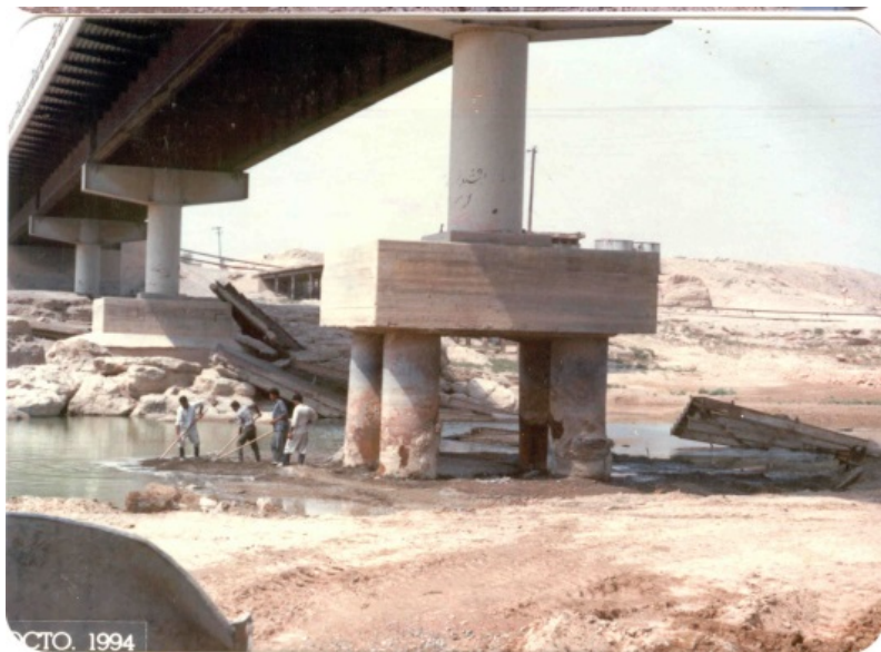
Figure 1.1 Bridge Scour in Iran (Institute for Hydromechanics (IfH), 1994)
