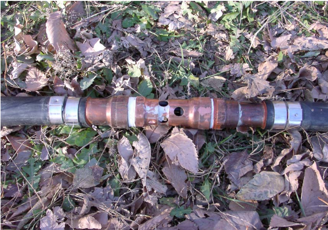
Figure 7 – Transducer port located between the straddle packers of the old receiver.
