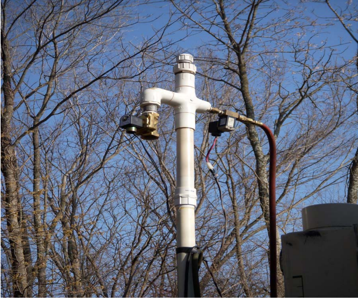
Figure 12 – Pneumatic air manifold.
