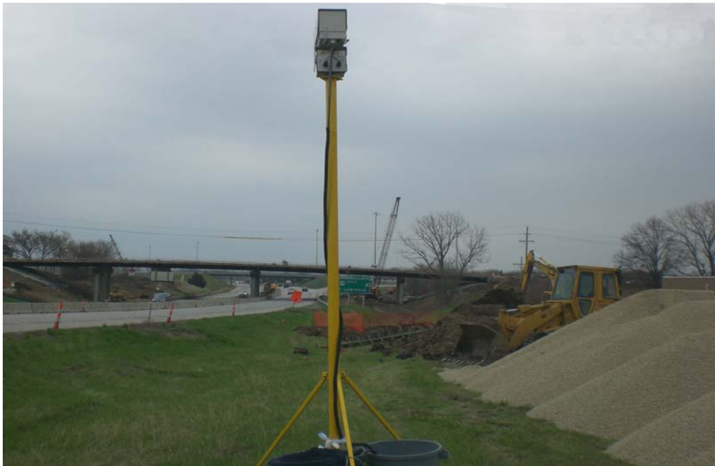
Figure 3. An on-site mounted video camera
