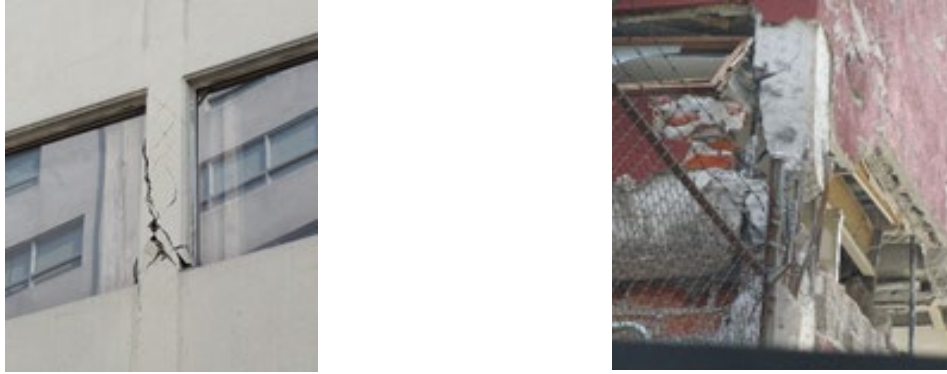
Figure 3. Examples of structural damage in buildings surveyed by CICM and SMIE (2017) (COLOR)
