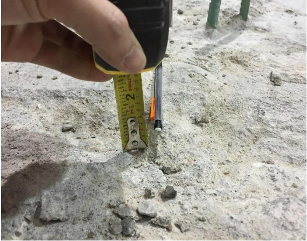
(a) Girder #1: Crater in girder top flange
