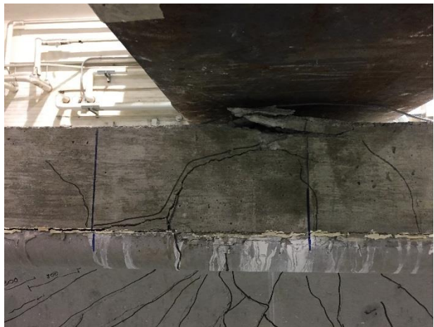
(d) Compression zone failure (Girder #2, but also similar to the failure of Girder #3)
