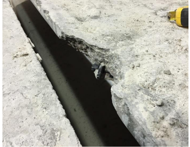
(b) Girder #3: Broken flange tip
