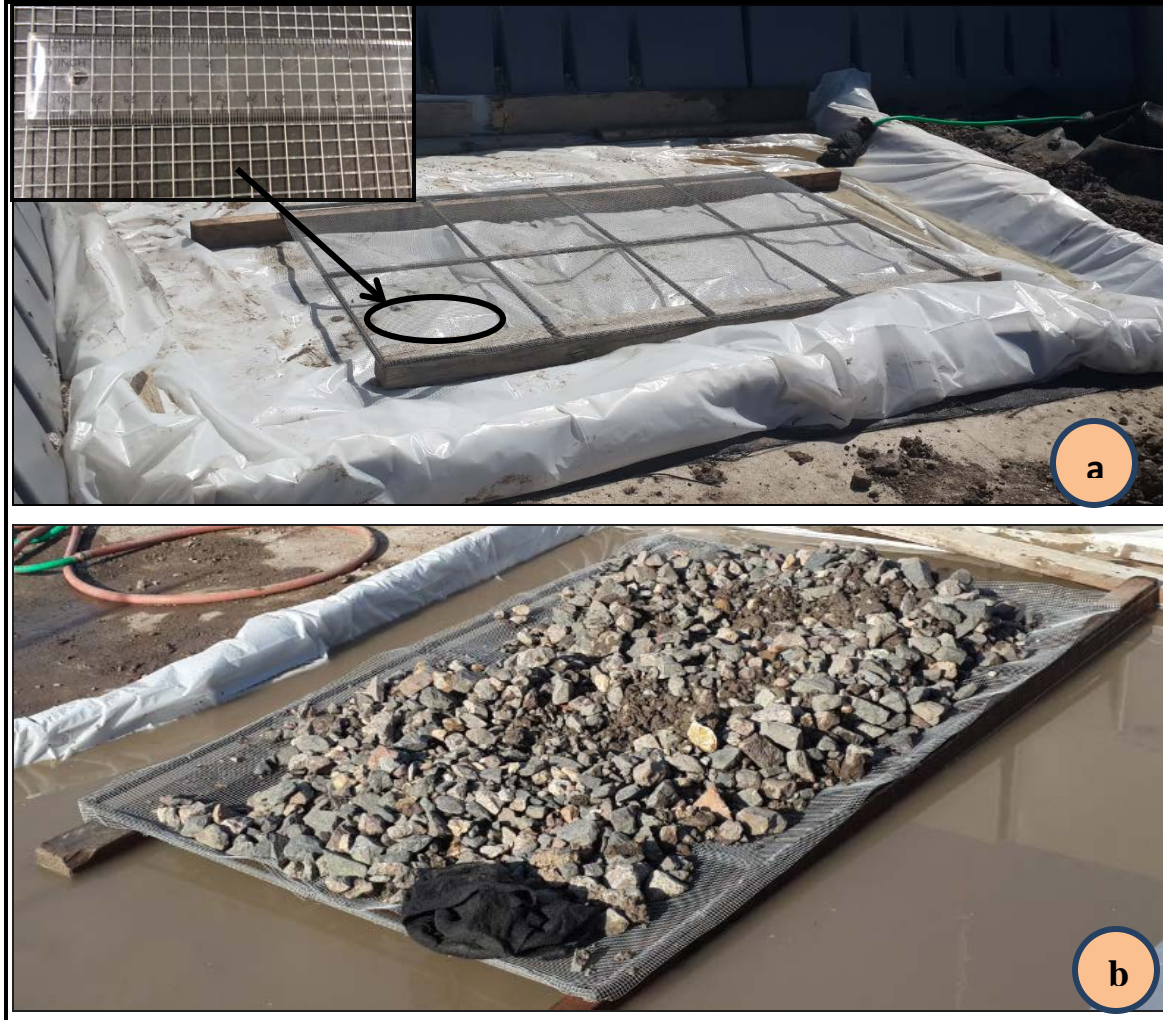
Figure 3-2 Ballast Recycling (a) Wire Sieve and Pond for Sieving (b) Sieving Procedure
