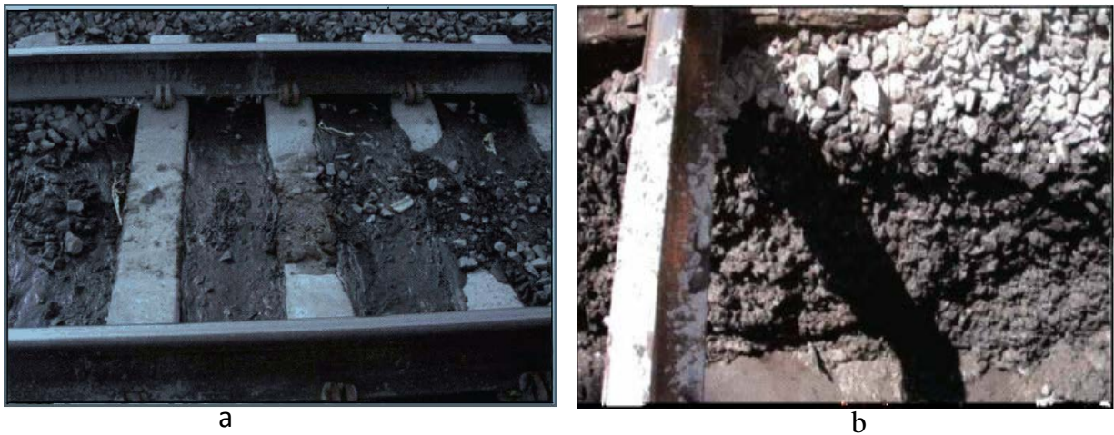
Figure 2-3 Fouled Ballast Layer after Pit Investigation (a) plan (b) section (Read et al. 2010)
