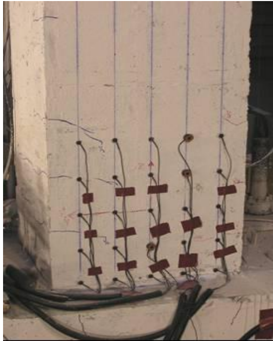
Figure 3.3: Crack pattern at bottom of Specimen 3 for a maximum drift ratio of 0.50%.
