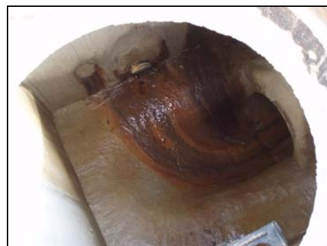
Photo 6. Inside of overflow structure showing drain pipe and orange biofilm.
