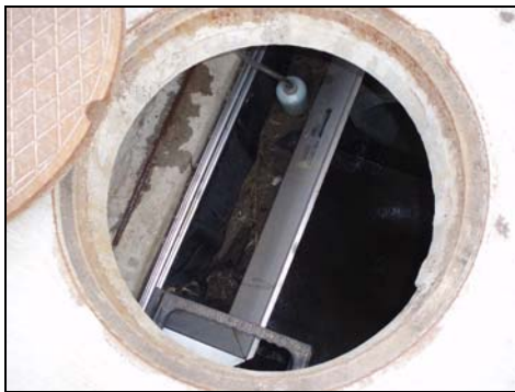
Photo 3. Mesh trap in storm sewer holding collection bottle.
