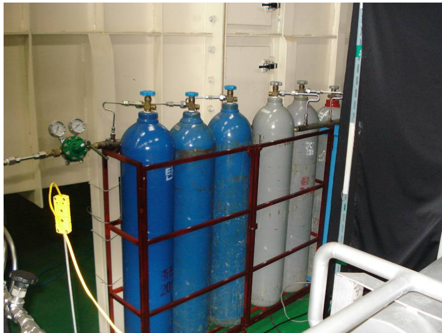
Figure 3.6 Pressure vessels of CO 2
