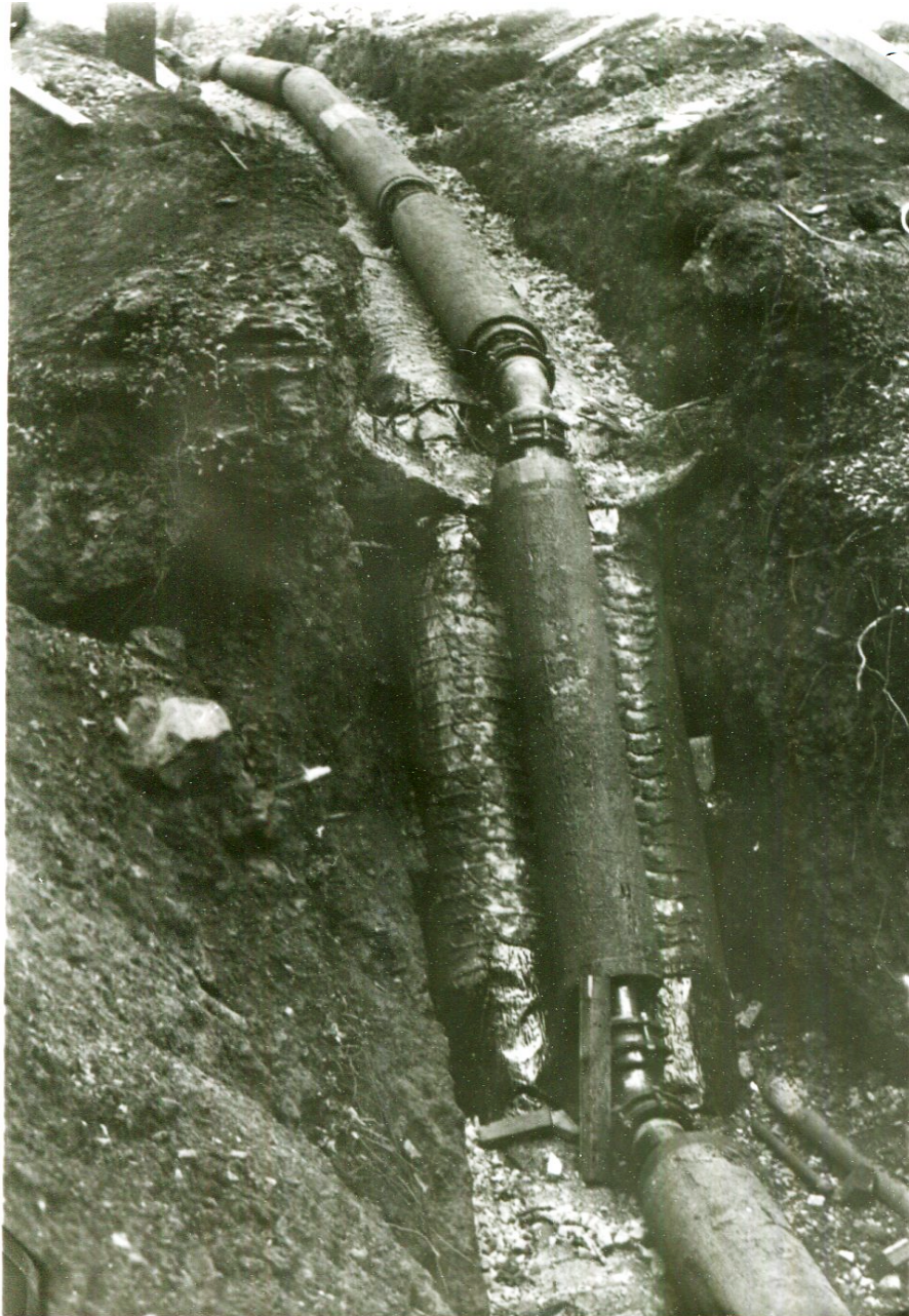
Fig. 5.6: Thermal water pipes for new collection and distribution system. These pipes traveled to the main line. Note the insulation around the pipes where none had originally appeared; HOSP 4544-52.
