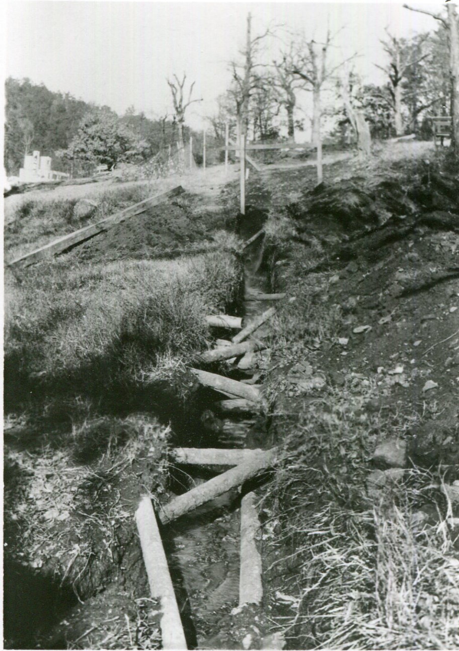
Fig. 5.5: The chaotic piping system from decades of improvements on Hot Springs Mountain, unearthed during the 1930-31 water collection and distribution overhaul project; Hamilton, Report of Construction of Hot Water Collecting and Distributing System , HOSP 4544-1.
