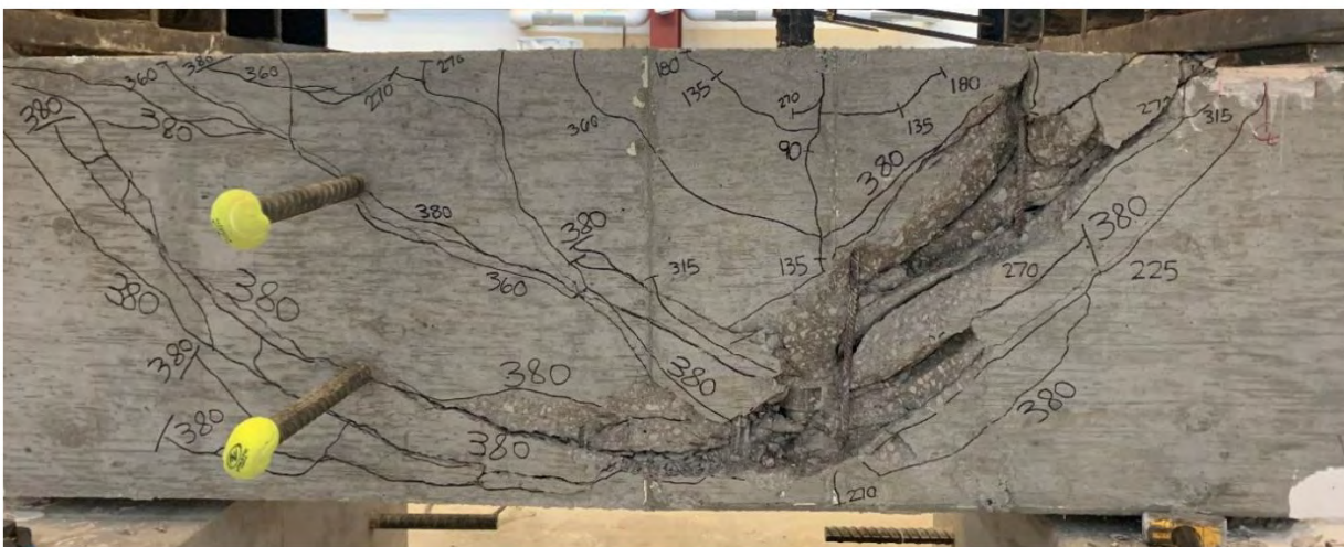
Figure 5.20 Anchorage failure observed in specimen 14-16B ( A_{tt}/A_{hs} = 0.178 ) tested under loading condition B
