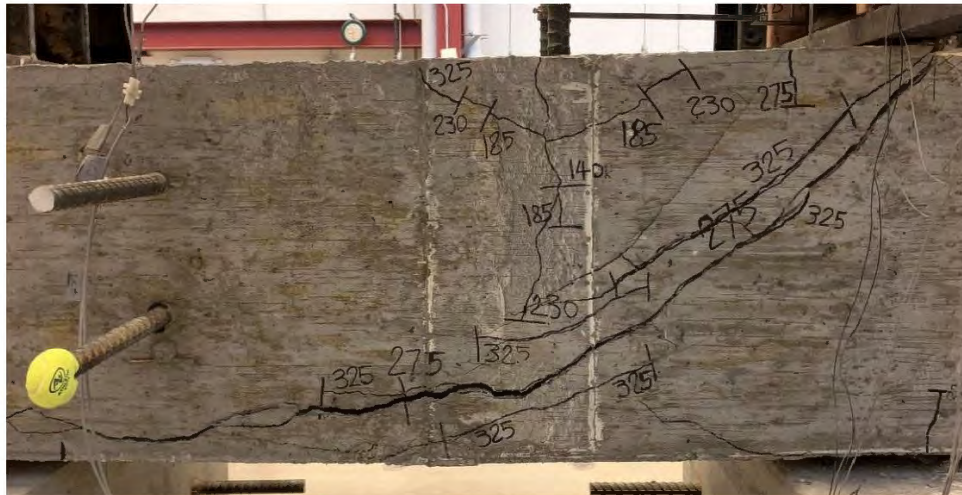
Figure 5.17 Shear-like failure observed in specimen 14-16A ( A_{tr}/A_{hs} = 0.178 ) tested under loading condition A
