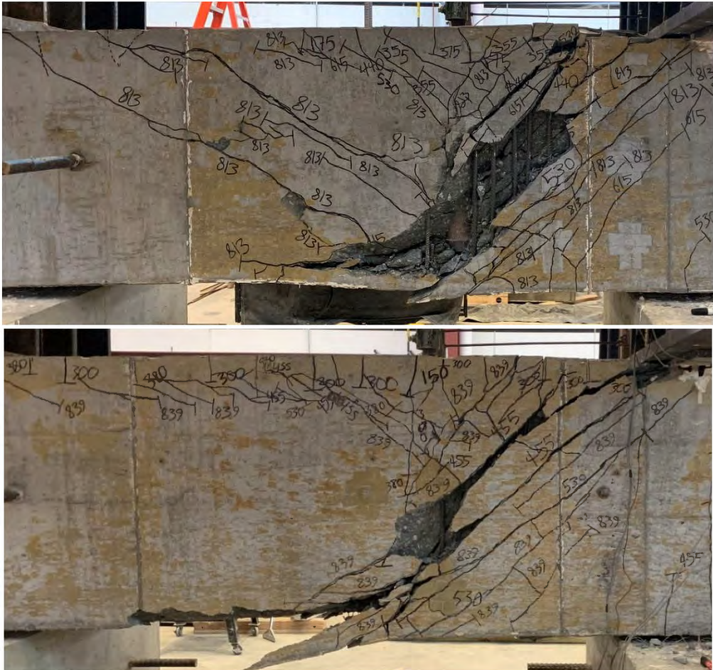
Figure 5.31 Comparing failure modes of specimen 18-2 with 3.5 in. side cover to the bar (top) with specimen 18-6 with 6.5 in. side cover to the bar (bottom), both with A_{tr}/A_{hs} = 0.543
