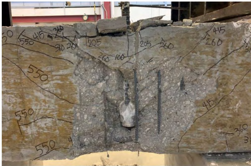
Figure 5.23 Anchorage failure observed in specimen 14-16D ( A_{tr}/A_{hs} = 0.827 ) tested under loading condition A (after removal of loose concrete)
