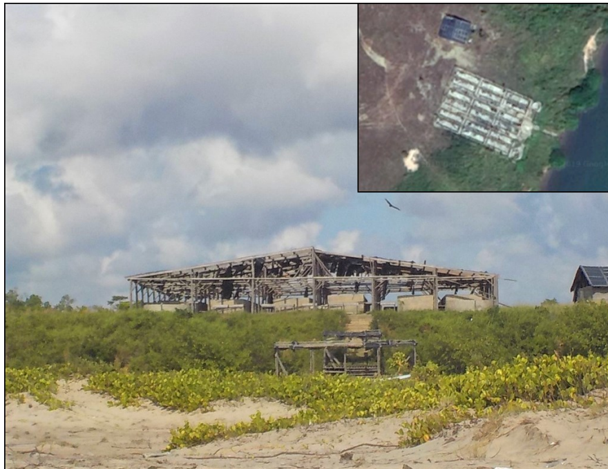
Figure 29: The Abandoned Río Ruk Ruk/ACASA JPF in November, 2017. The JPF was built by the processor ACASA in 2015, but it never operated (Source: Author, 2017; inset from Google Earth, 2019).
