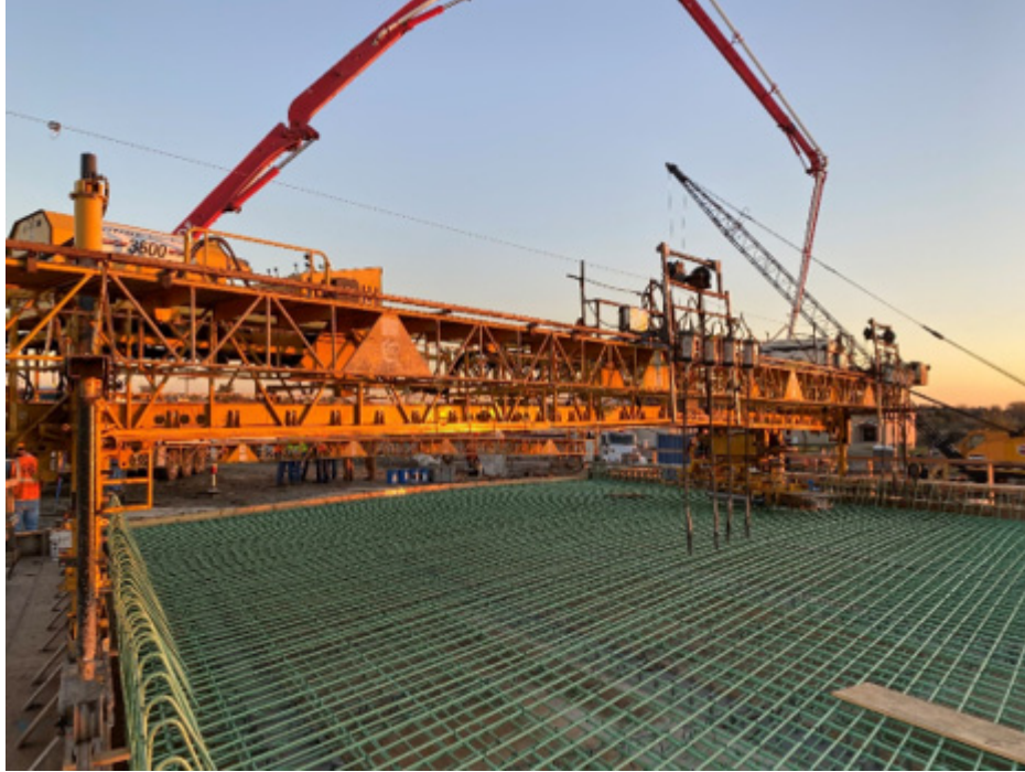
Figure 4.50: Consolidation and finishing equipment
