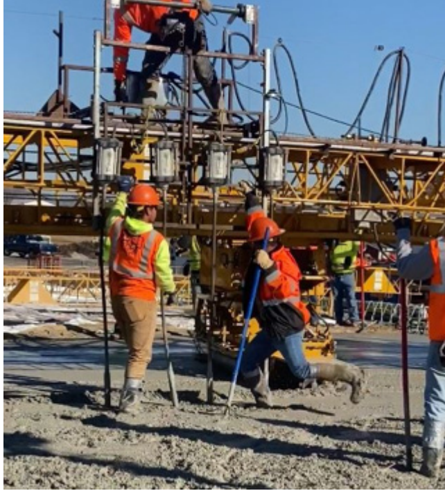
Figure 4.57: Malfunctioning of the machine-mounted gang vibrators
