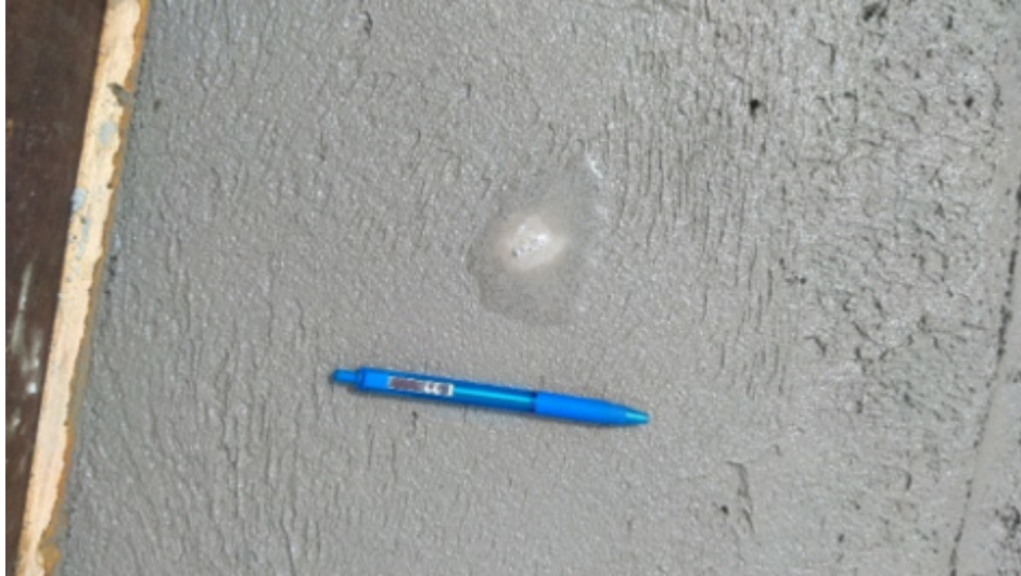
Figure 4.25: The appearance of air pockets on the concrete surface (image provided by MnDOT)
