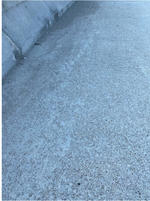
Figure 5.32: Scaling damage observed near the shoulders of KS-IC-LC-HPC-1
