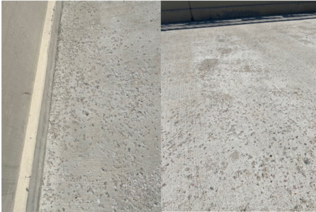
(a) (b) Figure 5.16: Scaling damage of MN-IC-LC-HPC-5 (a) near barriers; (b) a typical section for the remainder of the deck
