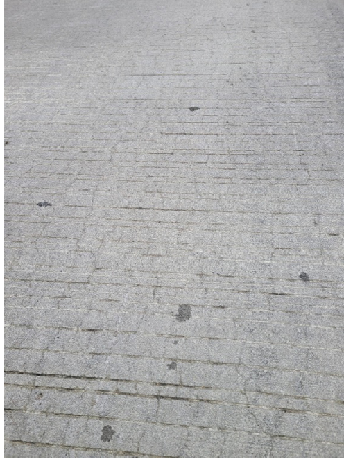
Figure 5.23: Map cracking on a typical section of MN-IC-LC-HPC-8
