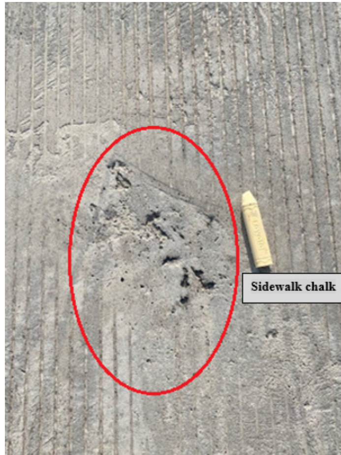
Figure 5.33: Surface damage observed on KS-IC-LC-HPC-2-P1
