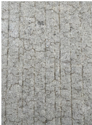
Figure 5.26: Map cracking on a typical section of MN-IC-LC-HPC-9
