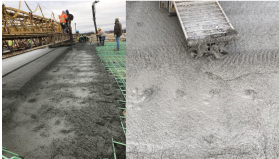
(a) (b) Figure 4.45: Holes left on the surface of the bridge deck. (a) overview; (b) close-up view
