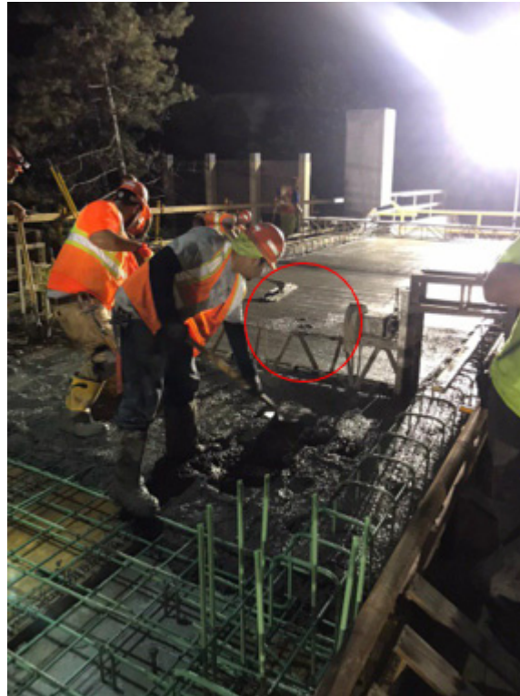
Figure 4.10: Holes in the concrete surface due to rapid removal of the spud vibrator
