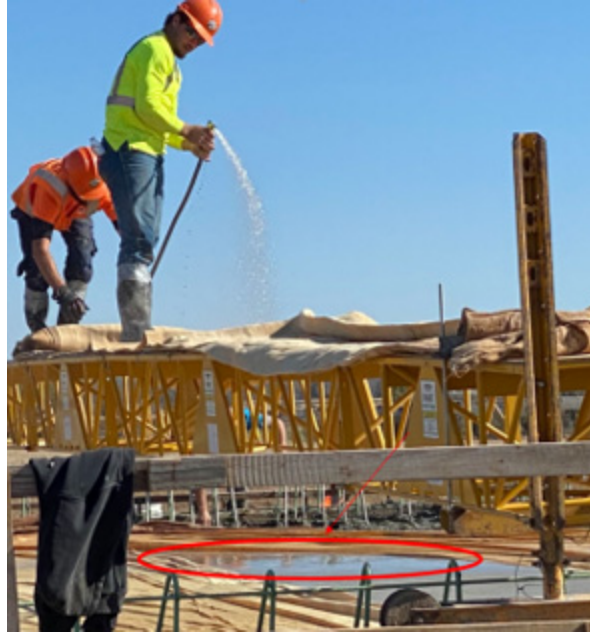
Figure 4.55: Ponding was observed on the deck
