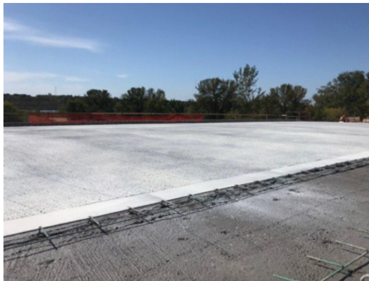
Figure 4.19: The application of the curing compound on the roadway of the deck
