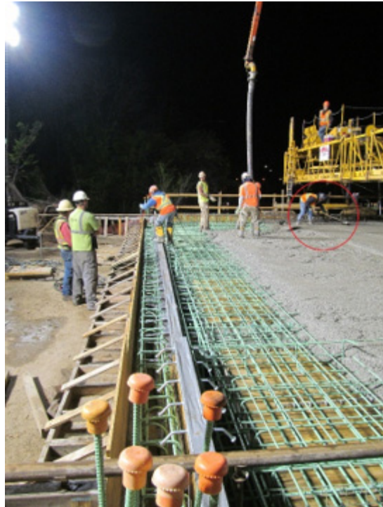
Figure 4.6: Disturbance of concrete observed near the north end
