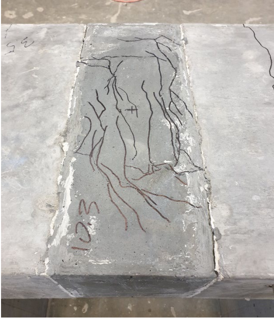
Figure 3.6: Splitting Cracks on the Top of UHPC Strip in Beam-Splice Specimen
