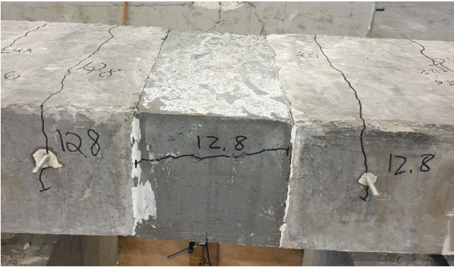
Figure 3.7: Splitting Crack on the Side of UHPC Strip in Beam-Splice Specimen
