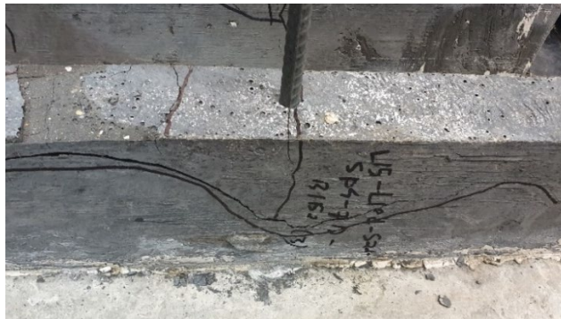
Figure 3.3: Open Diagonal Cracks on Pullout Specimen
