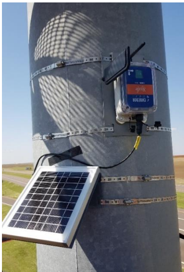
Figure 2-7 Xnode wireless sensor and solar panel
