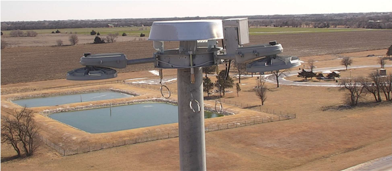
Figure 1: High Mast Illumination Pole Lighting Assembly with LED Luminaires (KDOT, 2019)
