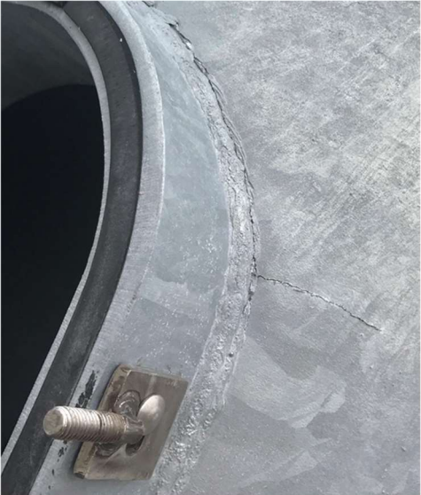
Figure 2: Cracking observed at the hand hole weld (KDOT, 2019)
