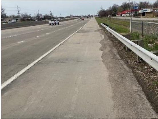
Figure 13: Dampness shown facing southbound direction near RP 217.55.
