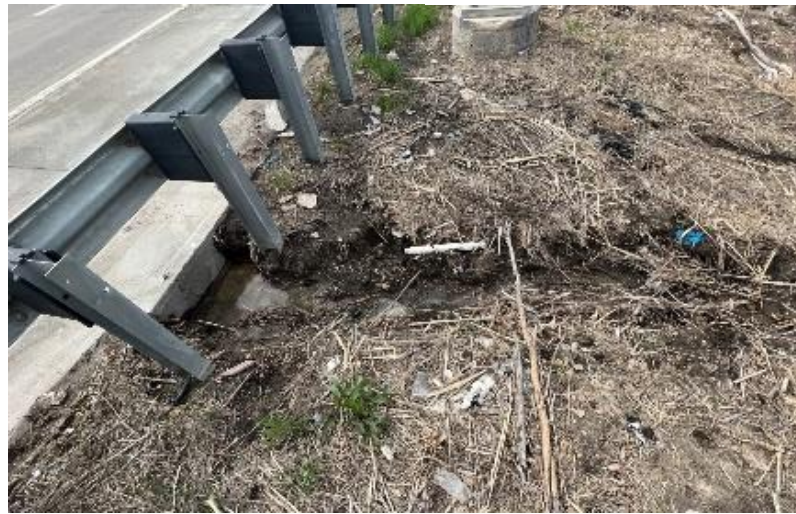
Figure 14: Washout near guardrail near RP 217.55.
