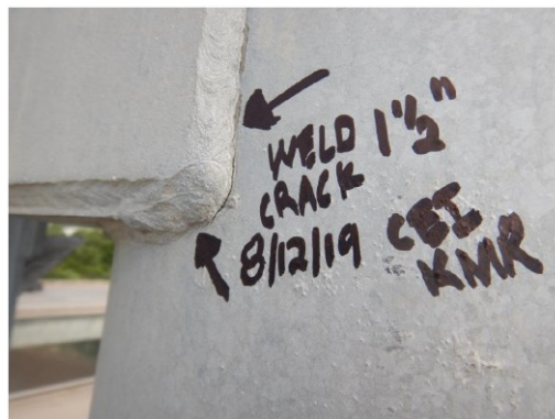
Figure 1.3. Cracking on COSS Box Connection (KDOT)
