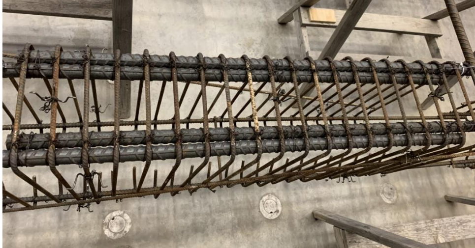
Figure 3.6: Heavily confined lap splice (14-g)
