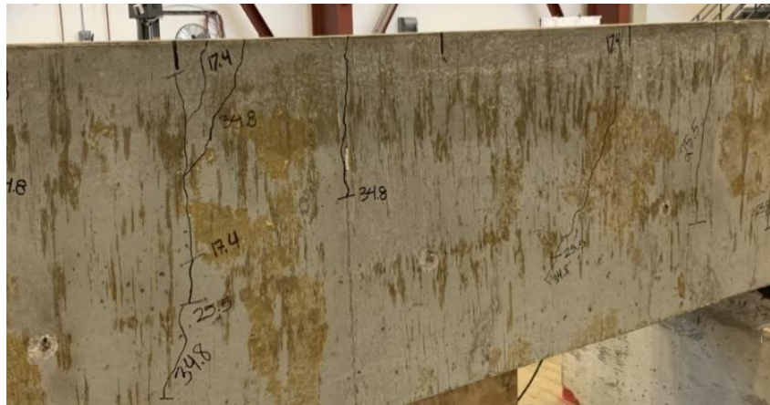
(b) Cracking during increased loading
