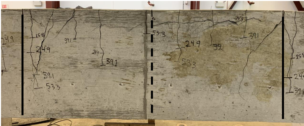
Figure E.8: Photo of 18-a after failure
