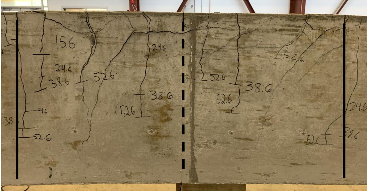
Figure E.9: Photo of 18-b after failure
