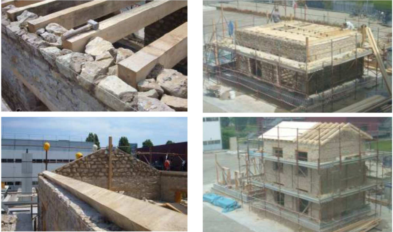
Fig. 6. Floor and roof details with details of wall connection (from Magenes et al. 2010)
