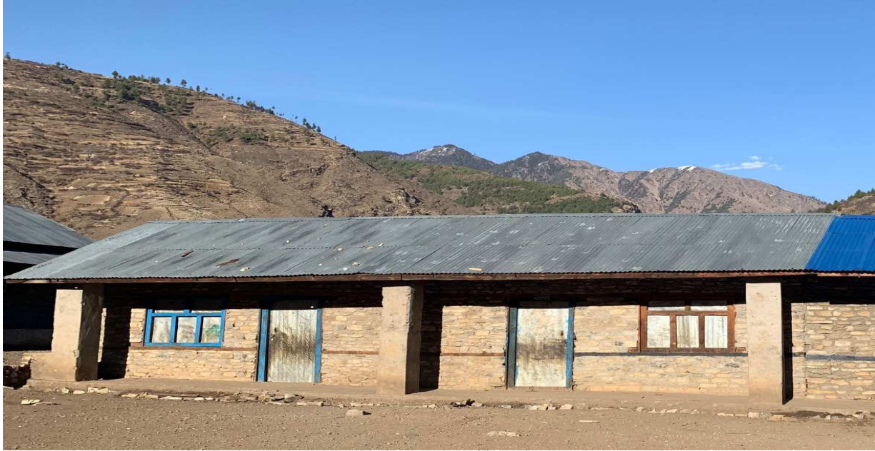
Fig. 2. Typical school building built with stone masonry walls in cement mortar with metal roof (Image credit: Dr. Elaina J. Sutley)
