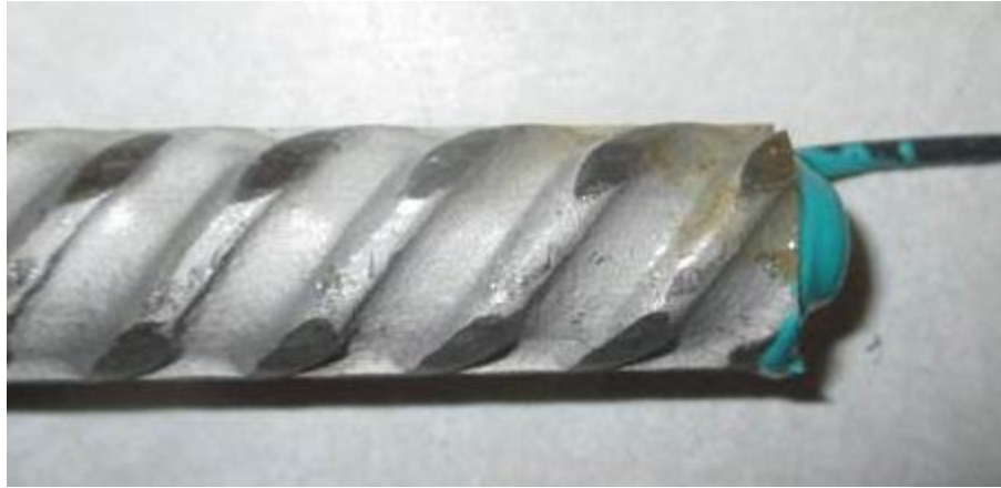
Figure 5: Closeup of corrosion on 2205 stainless steel reinforcement after one week of exposure to simulated seawater at 65 °F.
