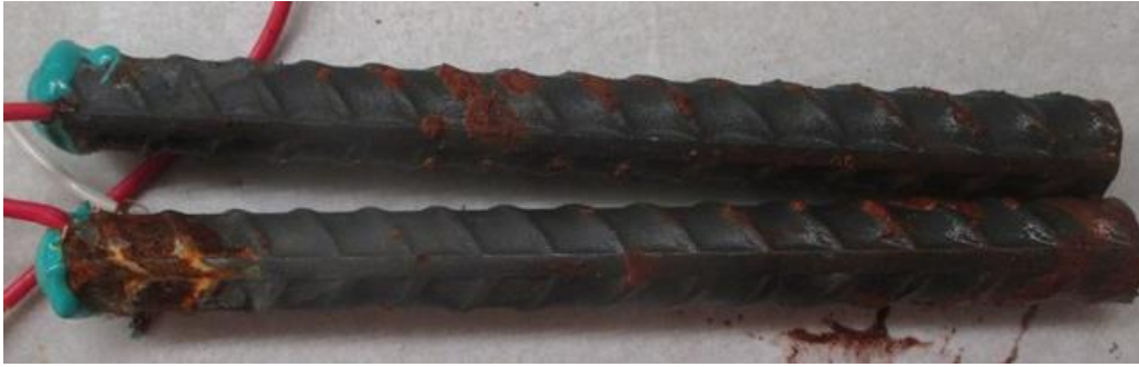
Figure 7: A1035-CS reinforcement after one week of exposure to simulated seawater at 65 °F.
