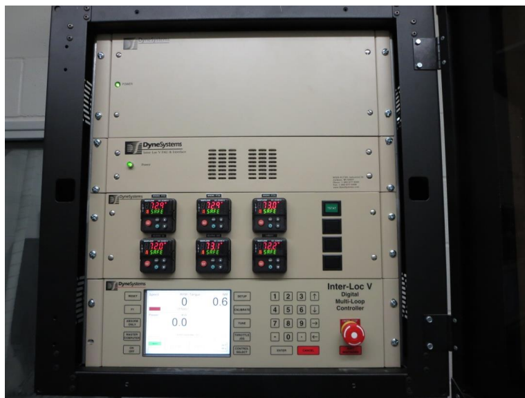
Figure C3. Dyne Inter-Loc V OCS, PAU, and CIA-III control and monitoring equipment.
