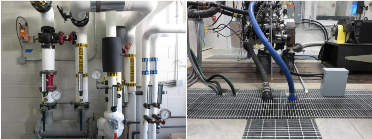
Figure C6. Fuel and coolant hardware interfacing with M2SEC building (left) and Duramax LBZ (right). The two segments interface with each other beneath the floor grates.
