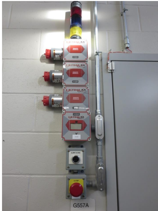
Figure C7. Multi-cylinder test cell gas and fire monitoring, emergency stop, and alarm systems.
