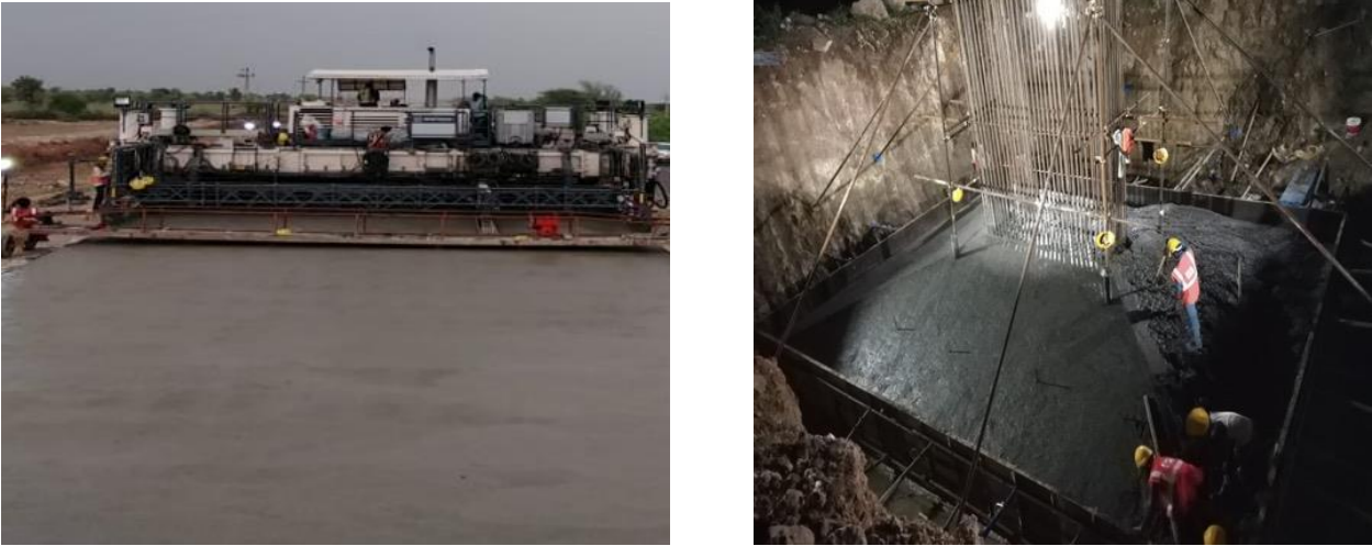
FIGURE 5.1. Progress Photos, Top left (PQC laying work in progress at Ch. 81.275 RHS) and Right (P6 raft concreting work).
