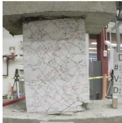
Figure C.4 – D80-1.5 at -4% chord rotation, second cycle
