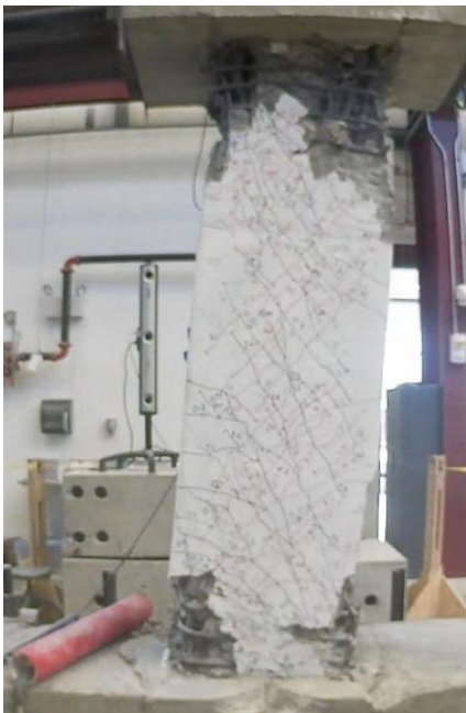
Figure C.54 – D80-3.5 at +8% chord rotation, second cycle
