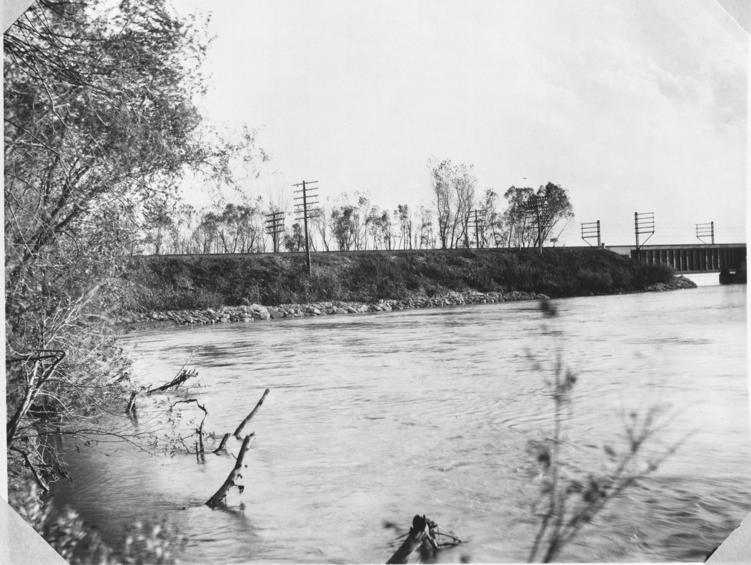
View No. 13 Line B Photo shows the flow of the Platte River against the railroad fill at the east end of the bridge. Line B adjacent to this fill.
