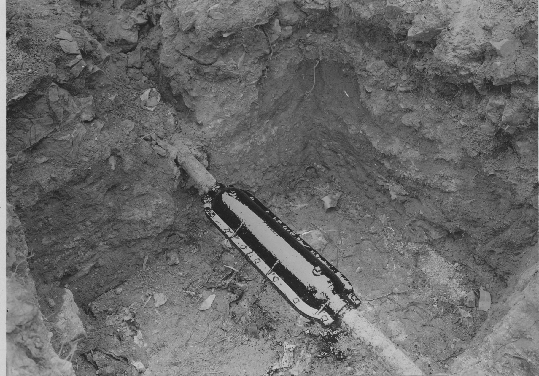
Figure 20. Cast Iron Splice Case on Tape Armored Cable.
