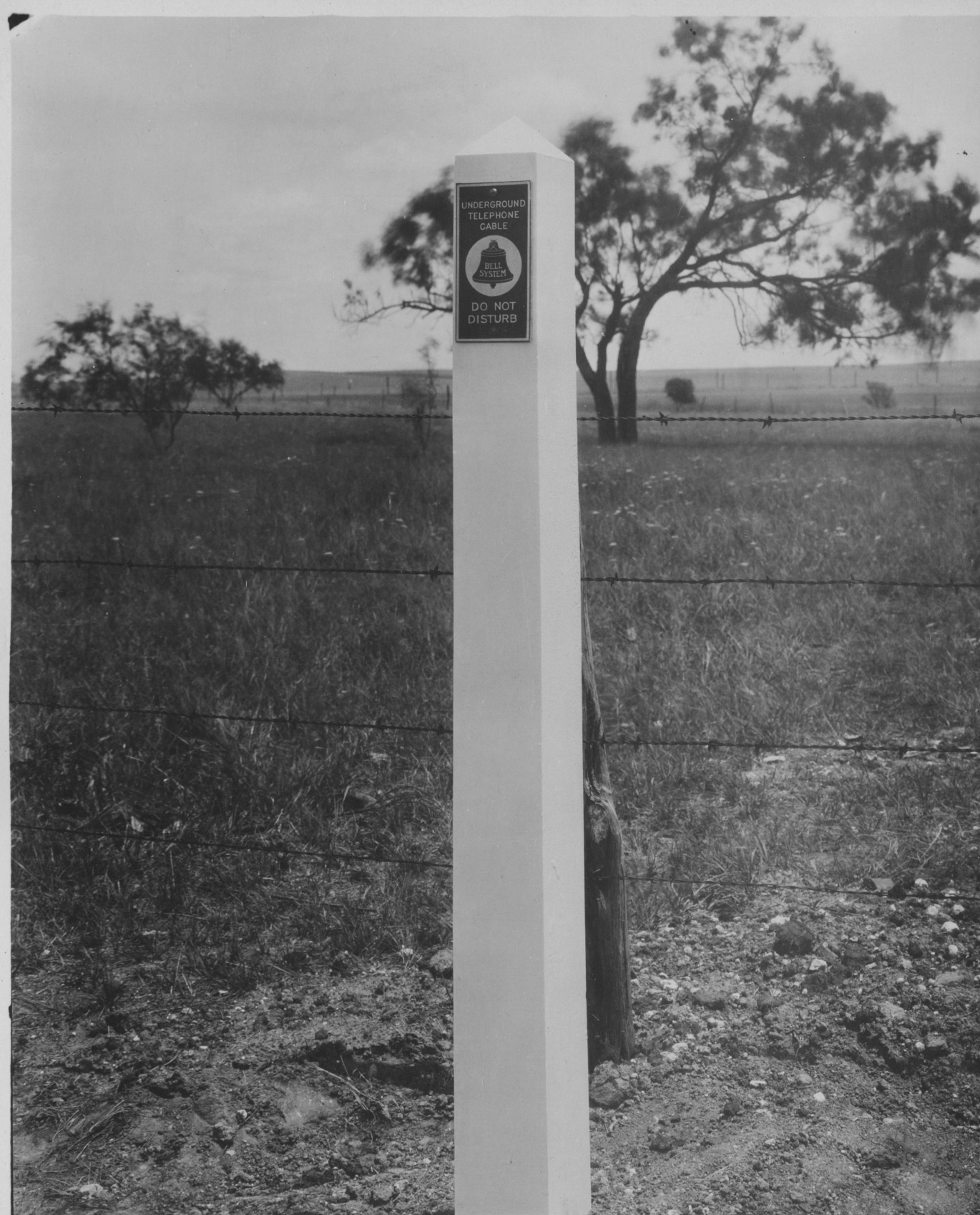
Figure 19. Warning Sign for Underground Cable.
