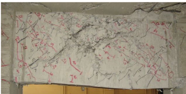
(b) Specimen CW-2: Reinforced Concrete (2 nd floor) beam, top, and HPFRC (4 th floor) beam, bottom
