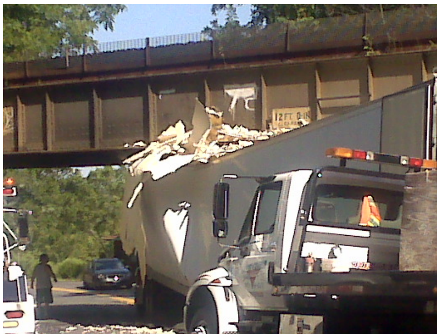
Figure 2-4: Tractor trailer collision resulting in a non-scheduled Damage Inspection to evaluate the structural integrity of the steel deck plate girder bridge. (Photo Credit: A. Elmore, NY)
