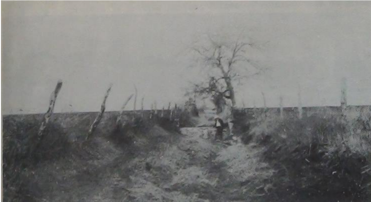
Figure 18: Farmers near Cleburne, Texas, used this former county road as a terrace outlet. Without proper protection from the increased runoff, it soon became a gully. Civilian Conservation Corps workers constructed the check dam pictured behind the man in the photo (ca. 1934) as a way to dampen the erosive power of runoff water. Source: Ellison, “Work of the E.C.W. Soil Erosion Camps in Alabama, Mississippi, Oklahoma and Texas,” 4a.
