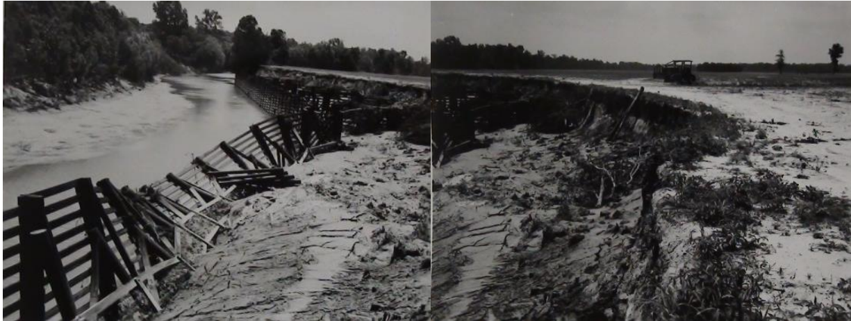
Figure 39: Streambank erosion along a stretch of Arkabutla Creek, ca. 1968. This bank eroded despite SCS bank-stabilization measures. Source: J. B. Furr and A. C. Allnutt, "Report of Investigation of Structure Failure, Arkabutla Creek Channel Bank Stabilization," 19 August 1968; b31; Item 213; RG 114; NACP.
