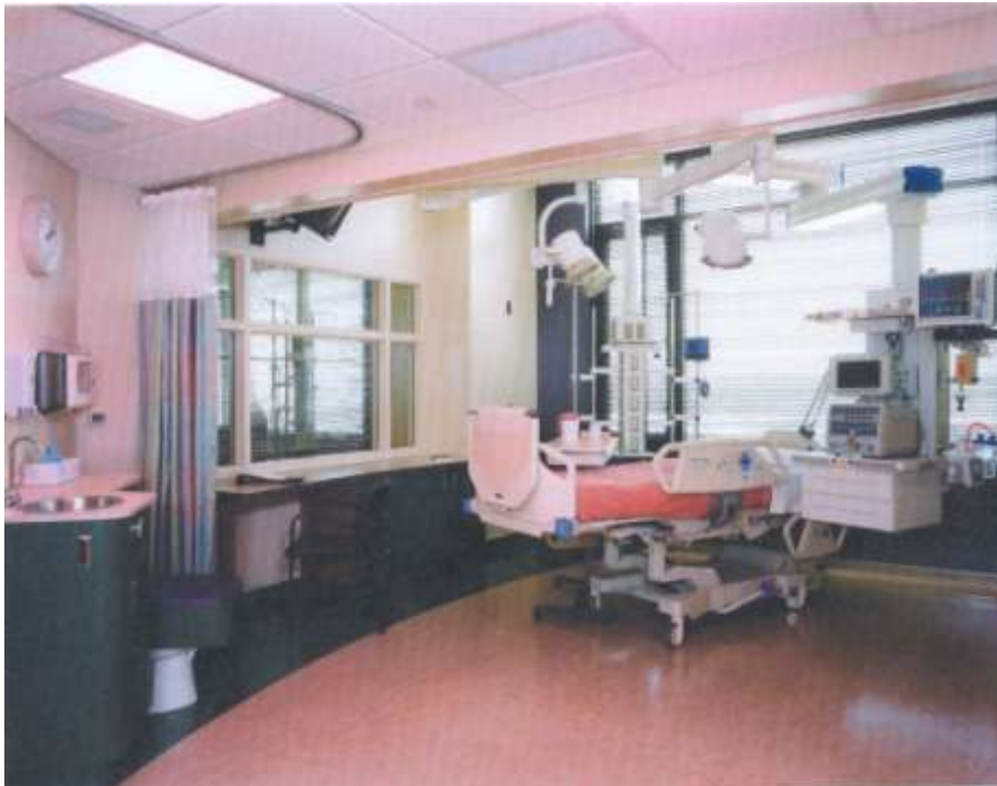
Figure 9: Ceiling-mounted boom in a patient room.
