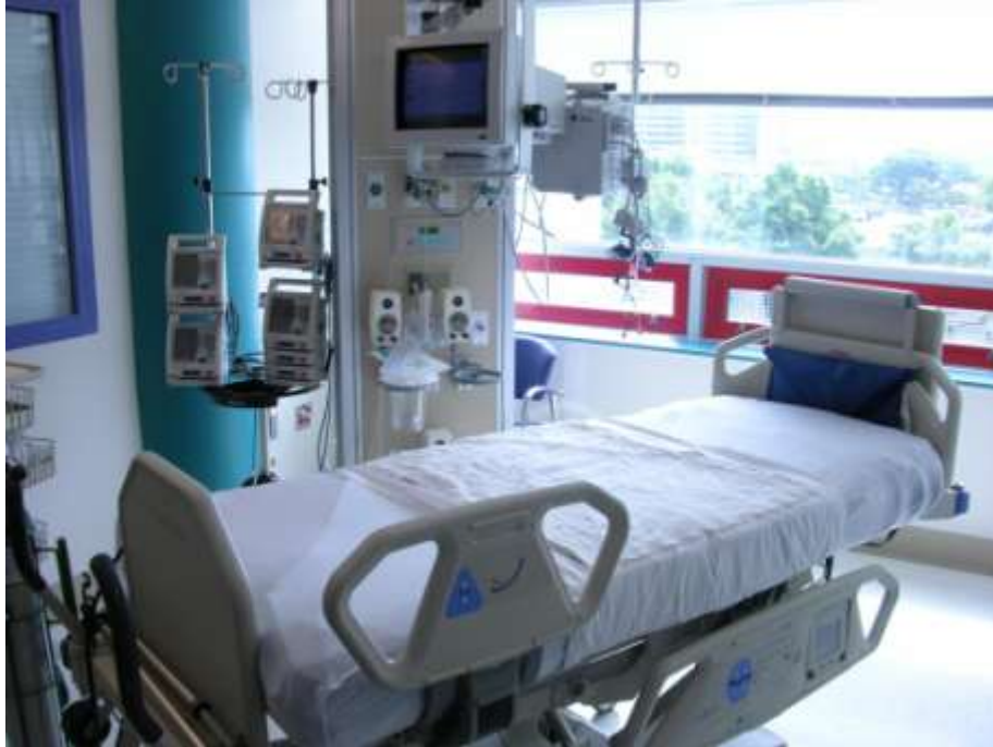
Figure 10: Power column in a patient room.
