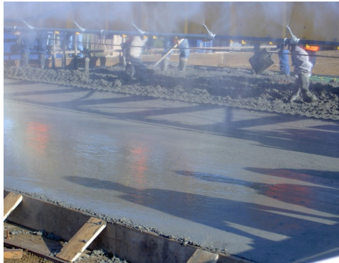
Figure 5.11 Fogging system deposited excessive water on slab – LC-HPC-8
