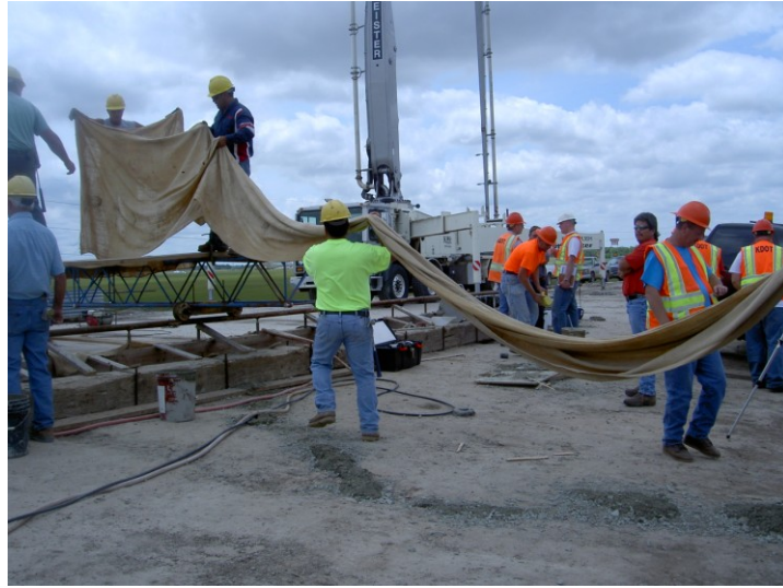
Figure 5.12 Improper use of areas near qualification slab for burlap placement – LC-HPC-11 qualification slab
