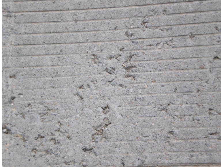
Figure 6.24 Improperly-sealed portions of deck surface – LC-HPC-3
