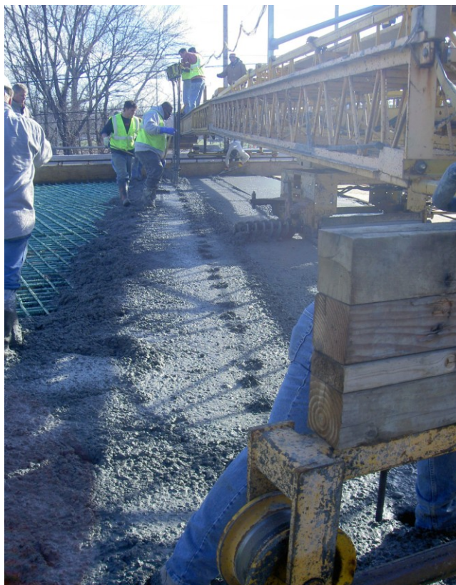
Figure 5.22 Holes left in concrete surface due to improper consolidation – OP Bridge Placement 1
