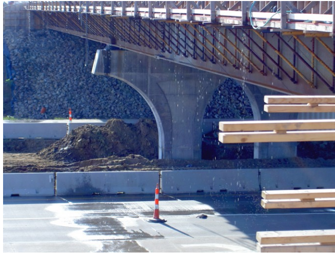
Figure 5.8 Water runoff due to over-wetting of the burlap – LC-HPC-7
