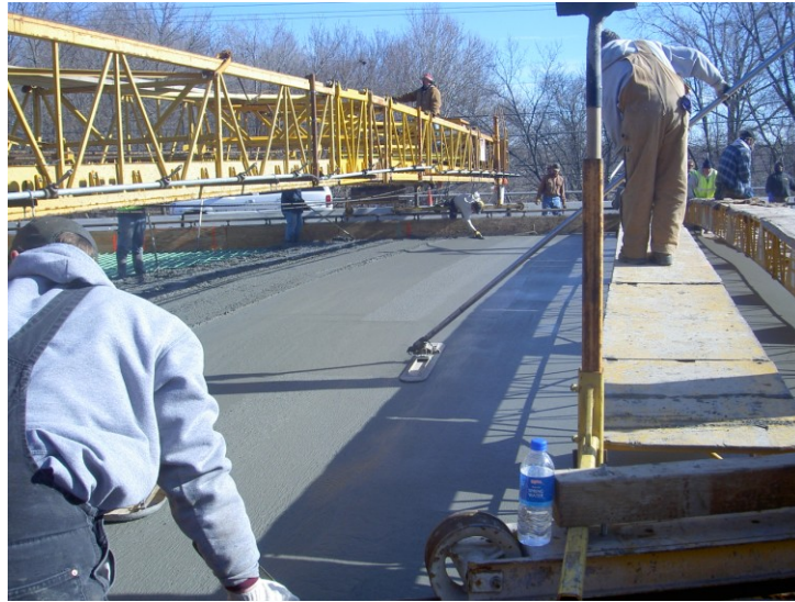
Figure 5.23 Bullfloating completed in longitudinal direction, perpendicular to work bridge – OP Bridge Placement 1
