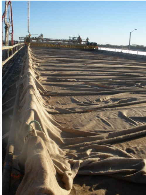
Figure 5.28 Burlap improperly tucked near barrier reinforcement – LC-HPC-16
