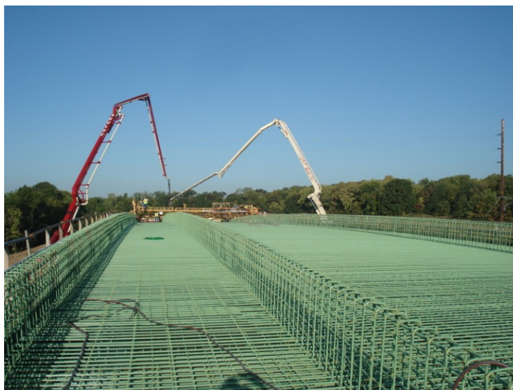
Figure 5.32 Barrier between recreational trail and roadway contributed delays in finishing and curing – LC-HPC-17
