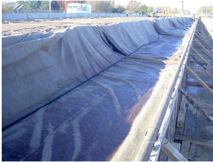
Figure 5.17 Burlap hung over barrier steel to minimize contact between burlap and sidewalk surface – LC-HPC-3
