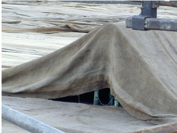
Figure 5.4 Burlap improperly tucked near barrier reinforcement – LC-HPC-2 qualification slab
