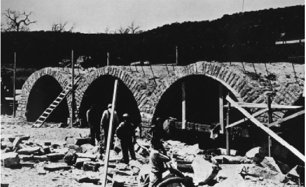
10. WPA masons building the Brazos River Bridge, Palo Pinto County, Texas, 1940 (photo: courtesy of the Texas Department of Transportation)
