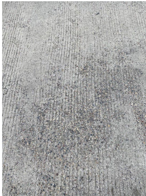
Figure 3.2: Scaling damage of bridge 27W06
