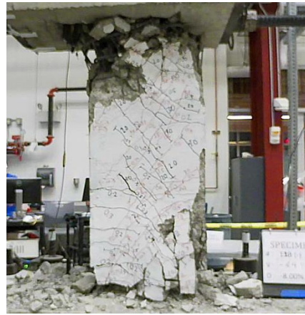
Figure C.39 – D80-2.5 at -10% chord rotation, first cycle
