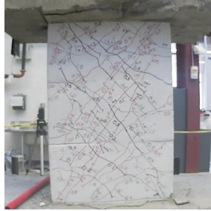
Figure C.10 – D100-1.5 at -2% chord rotation, second cycle
