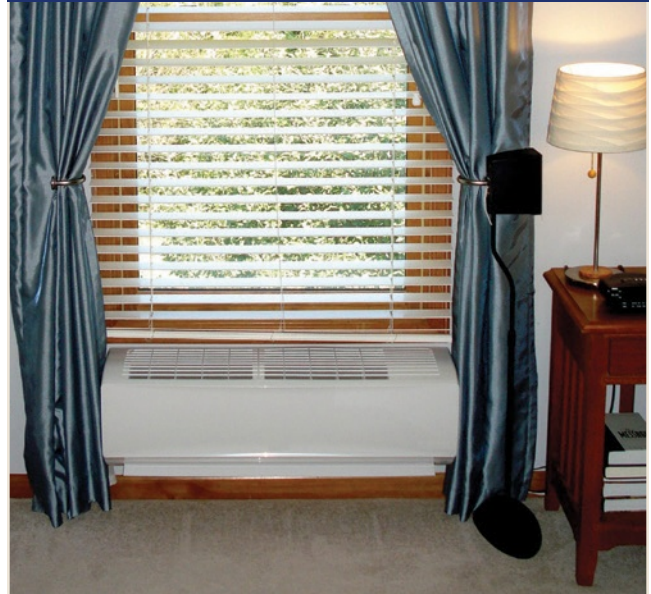
PHOTO 4 The indoor unit of the mini-split system was installed, by necessity, low-sidewall rather than high. Its discharge, at the bottom, was set to throw air down the hallway just opposite this window. In cooling mode a thin, very cold but dehumidified layer of air is produced; no moisture condensation occurs on the thicker-type carpet and pad.
