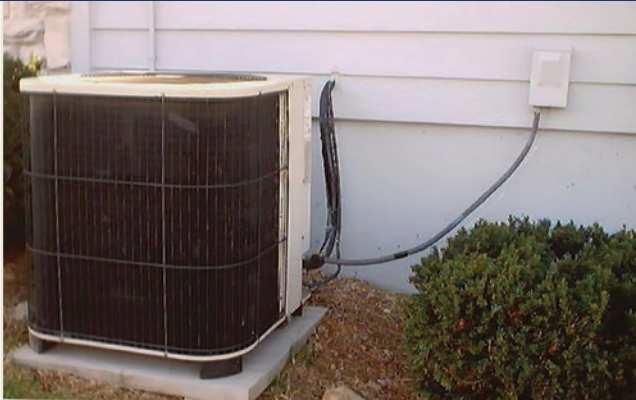
PHOTO 1 The original four ton (14 kW), SEER 10, R-22 condensing unit that had settled several inches, stressing its line set. Note the easy to inspect and clean fins it had.
