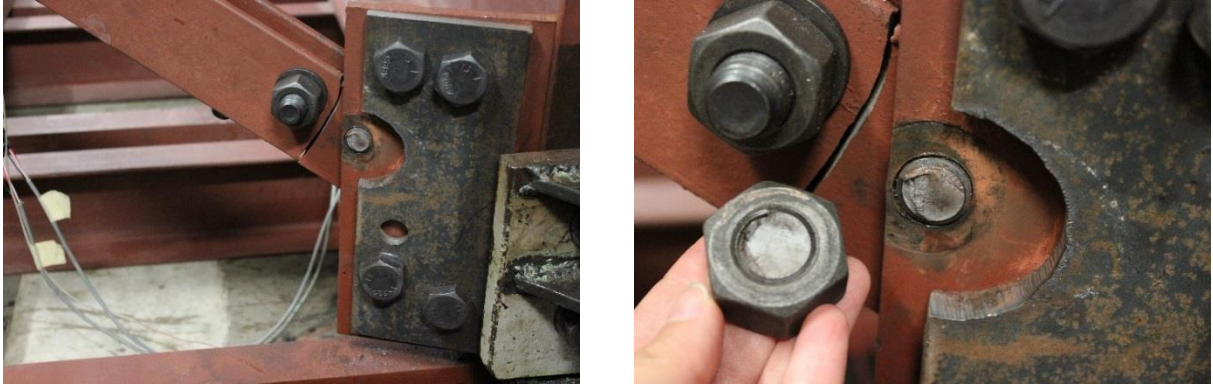
Figure 3-4: Shear failure of the bolt connecting the steel angle and cross-frame
