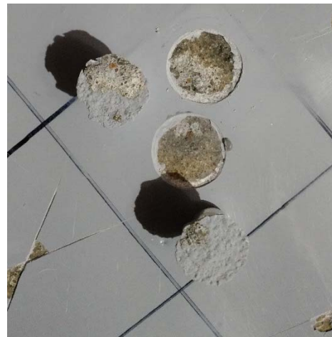
Figure 2.10: Pull-off test exhibiting coating and partial coating failures
