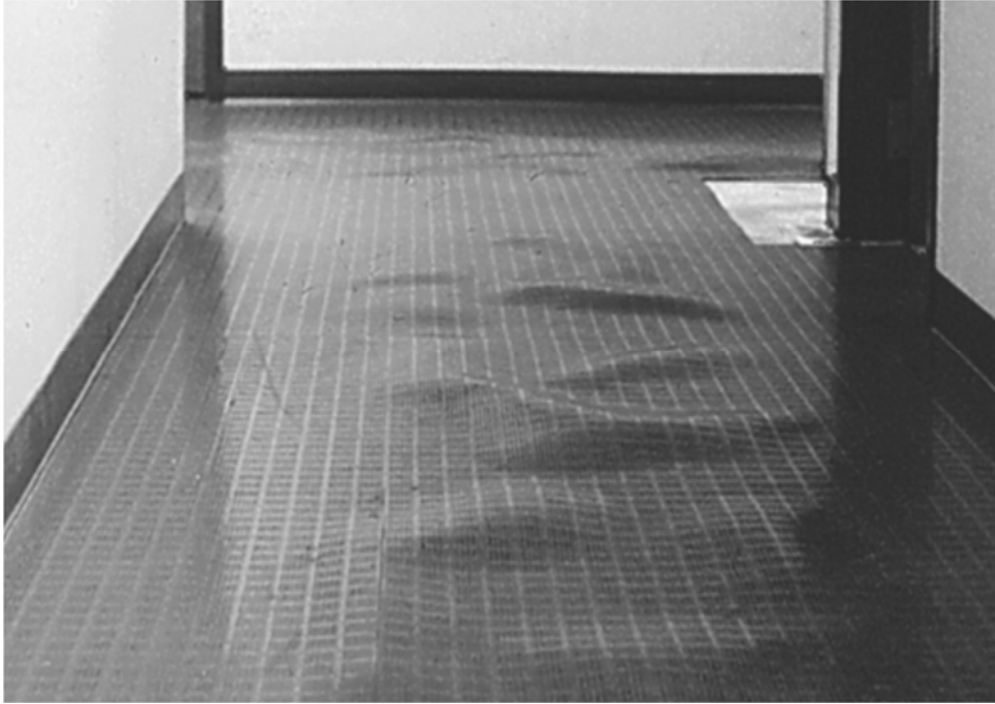
Figure 1.3: Debonding of floor covering (ACI 302.2R-06)
