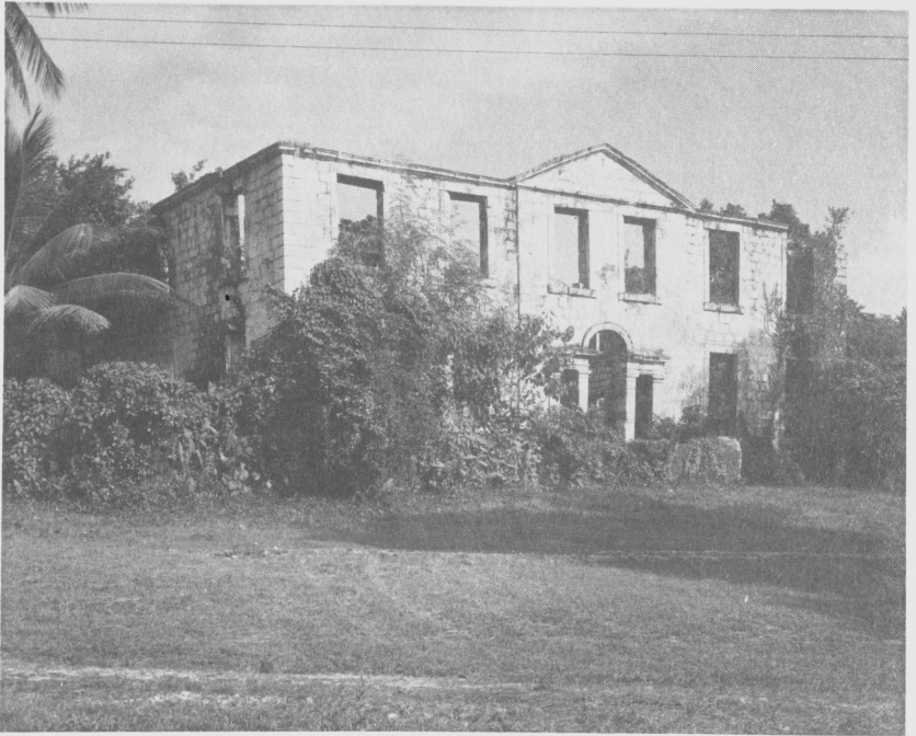
Figure 10.3. Good Hope estate hospital, Jamaica. Photographed in 1974 by Mr. P. J. Hanbury Tenison of Good Hope estate.
