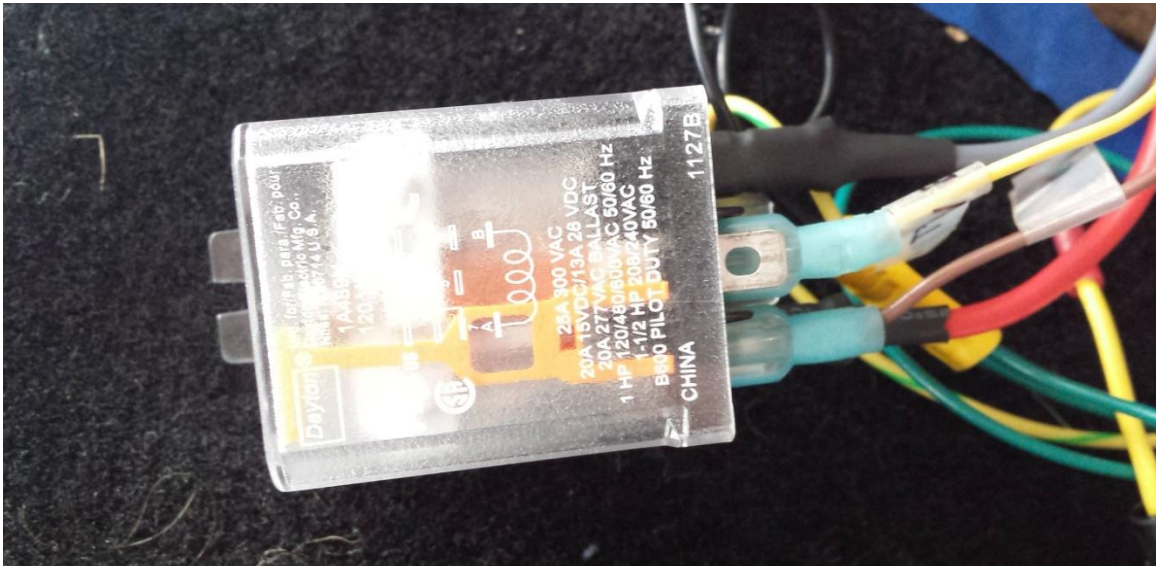
Figure 140: The ice cube relay provides the BMS with 12 VDC power when an AC power source is present. This ensures that the BMS can actively balance cells as needed.
