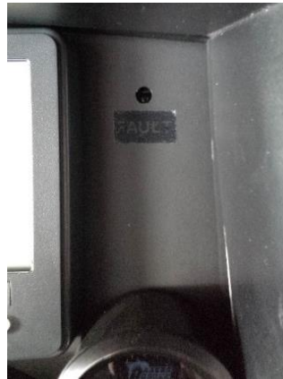
Figure 101: The fault light is located on the dashboard above the 12 VDC gauge.
