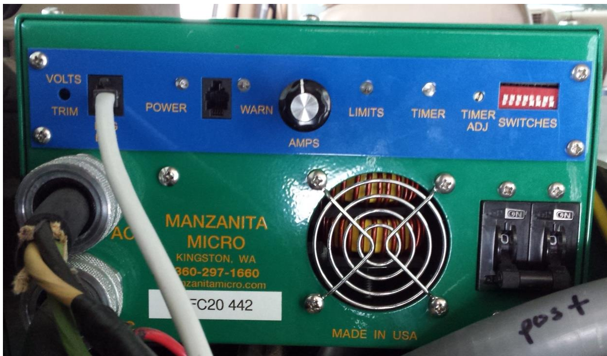
Figure 136: Manzanita Micro PFC-20 charger operating panel
