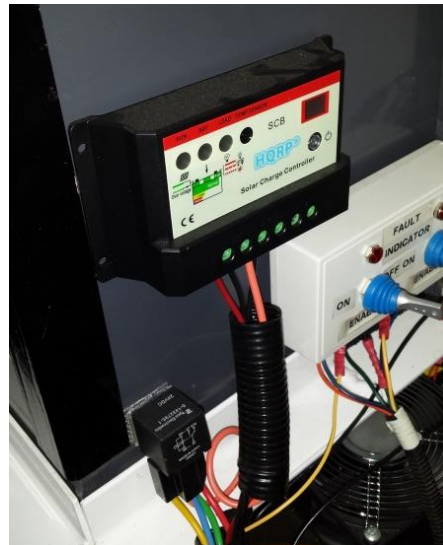
Figure 153: HQR solar controller and system relay.
