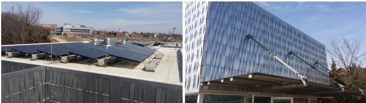
Figure 185: The Hill Engineering Research and Development Center solar arrays. The roof panels (left) provide 11.7 kW, and the front awning (right) provides 3.1 kW.
