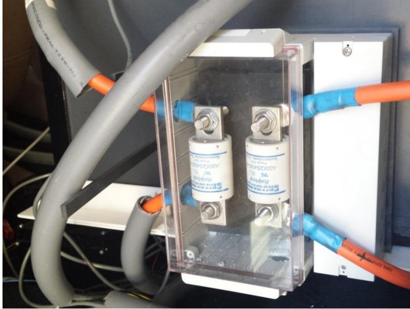
Figure 106: The HV fuses are located inside the driver's side passenger door.
