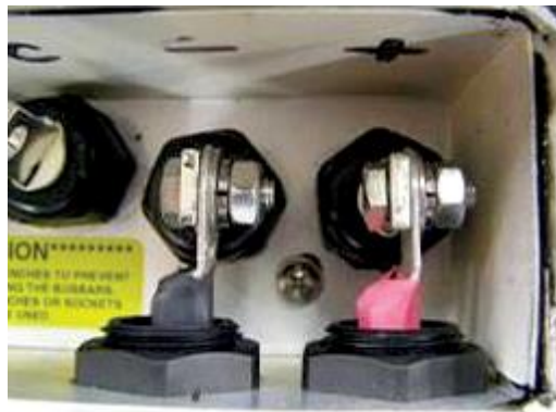
Figure 28: High voltage connections for the DMOC445 [24].
