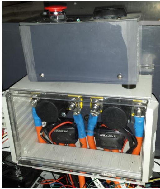
Figure 107: HV junction box illustrating the two contactors (top) and two junction blocks (bottom).
