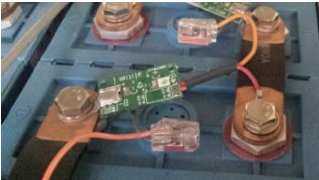
Figure 110: The BMS cell boards are installed between the positive (right) and negative terminal (left) of each cell.
