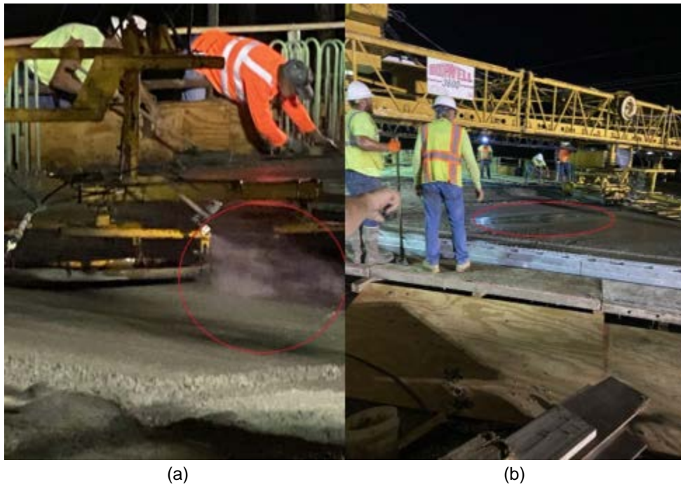
Figure 2.64: Excessive Water on the Deck (a) Unadjusted Nozzles; (b) Ponded Water on the Surface
