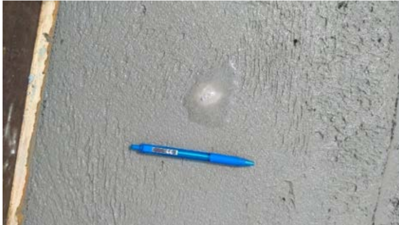
Figure 2.26: The Appearance of Air Pockets on the Concrete Surface (Image Provided by MnDOT)
