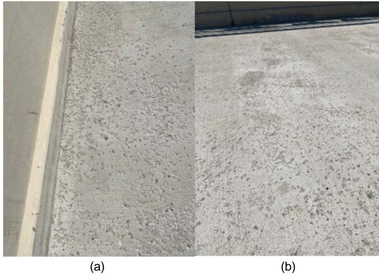
Figure 3.16: Scaling Damage of MN-IC-LC-HPC-5 (a) Near Barriers; (b) A Typical Section for the Remainder of the Deck
