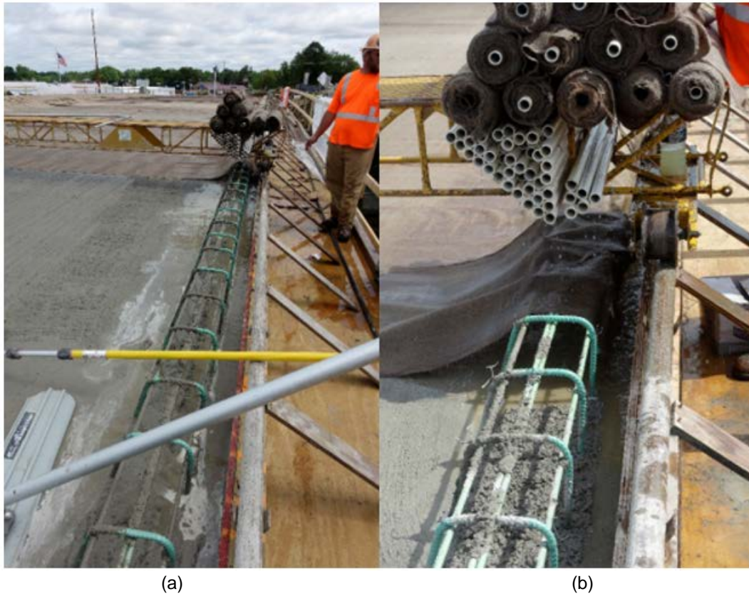
Figure 2.6: Water from Burlap Dripping onto the Deck (a) An Overview; (b) A Close-Up View
