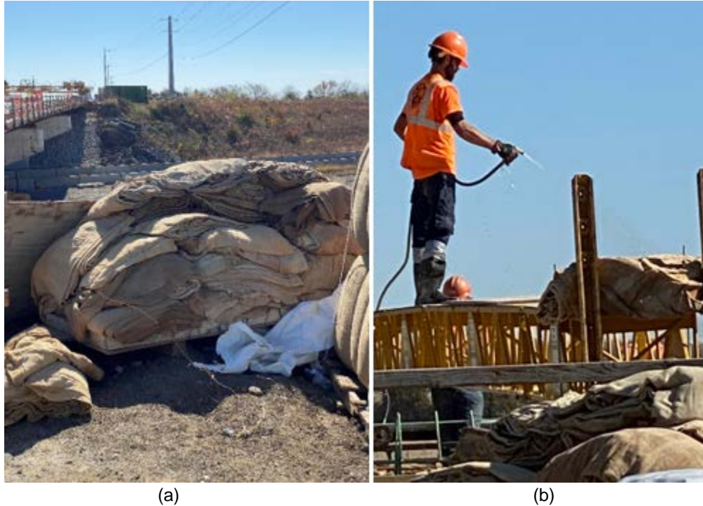
Figure 2.54: Burlap Placement of KS-IC-LC-HPC-2 (a) Dry Burlap; (b) Wetting the Burlap on the Deck
