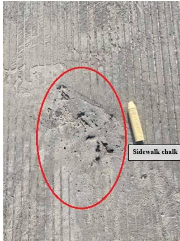
Figure 3.34: Surface Damage Observed on KS-IC-LC-HPC-2-P1
