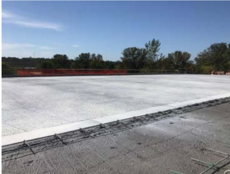
Figure 2.20: The Application of the Curing Compound on the Roadway of the Deck Showing Uneven Coverage
