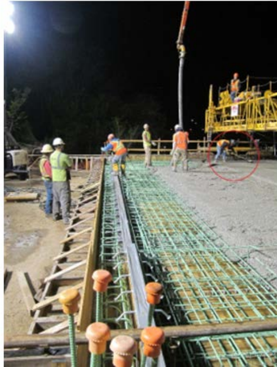
Figure 2.7: Disturbance of Concrete Observed Near the North End
