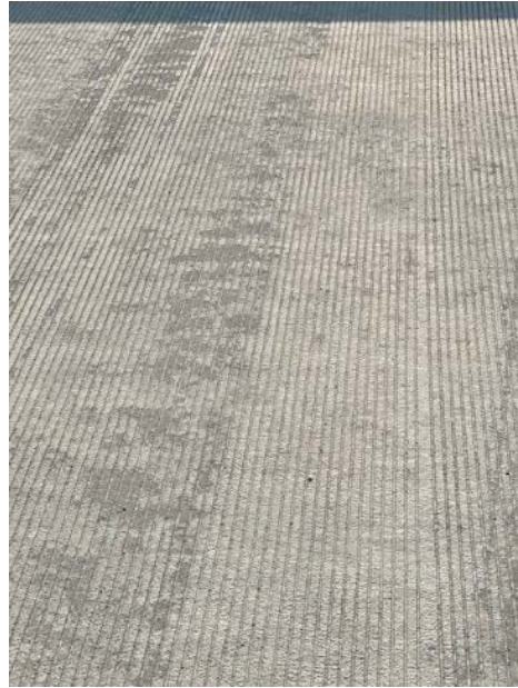
Figure 3.38: Scaling Damage Observed on Some Portions of KS-IC-LC-HPC-2
