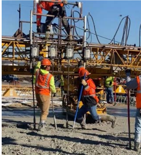
Figure 2.57: Malfunctioning of the Machine-Mounted Gang Vibrators
