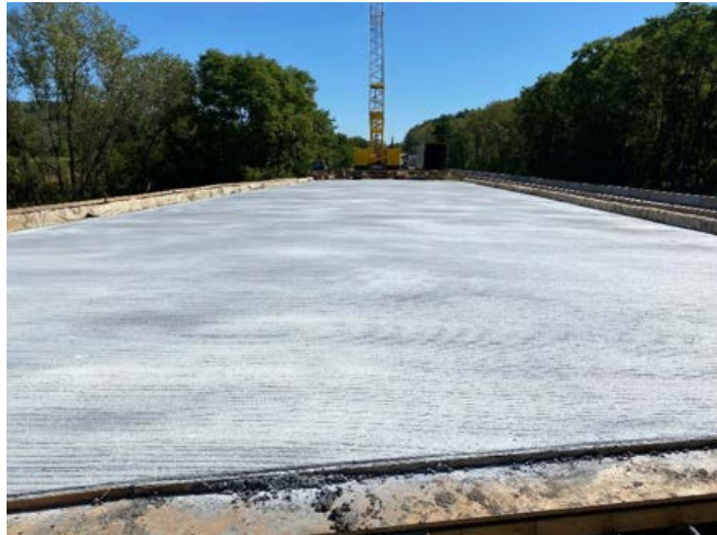
Figure 2.37: Non-Uniform Application of the Curing Compound on the Deck
