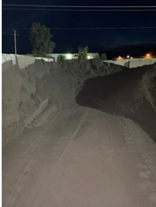
Figure 4.34: Disturbance of the bottom of the stockpile
