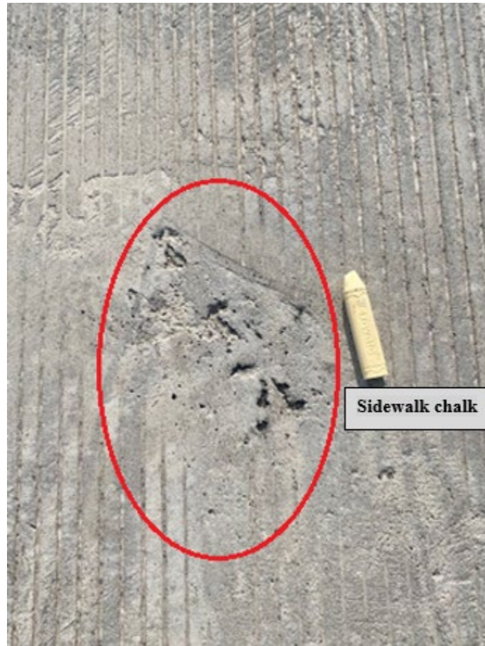
Figure 5.33: Surface damage observed on KS-IC-LC-HPC-2-P1
