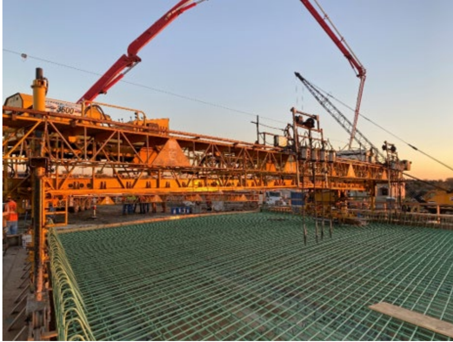
Figure 4.50: Consolidation and finishing equipment
