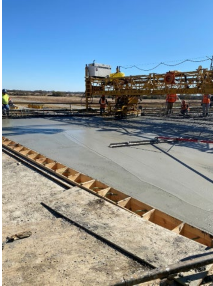
Figure 4.53: Overfinishing the deck in the presence of bleed water
