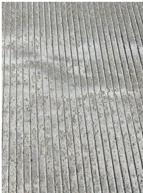
Figure 5.38: Scaling damage observed on some portions of KS-IC-LC-HPC-3
