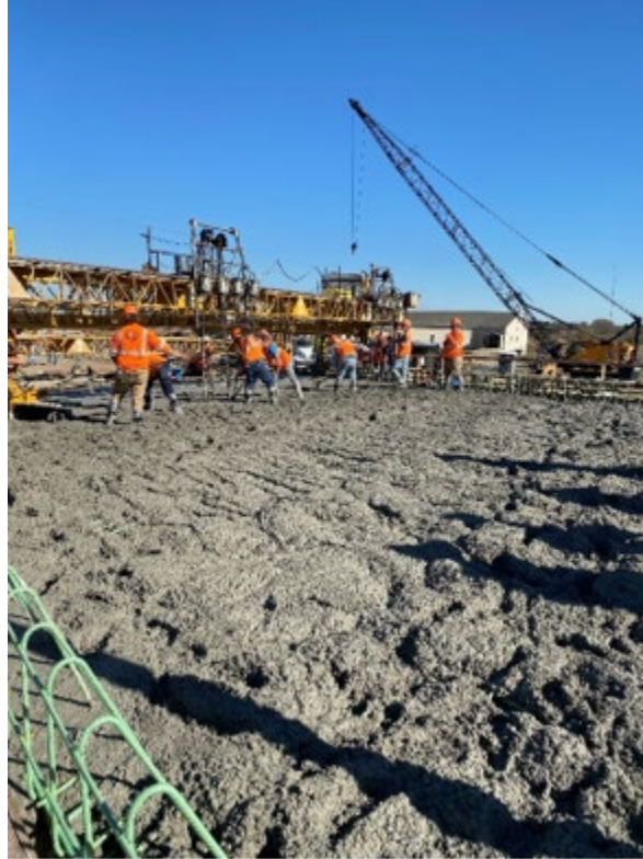
Figure 4.52: Concrete was left unconsolidated and unprotected due to inoperable roller screed
