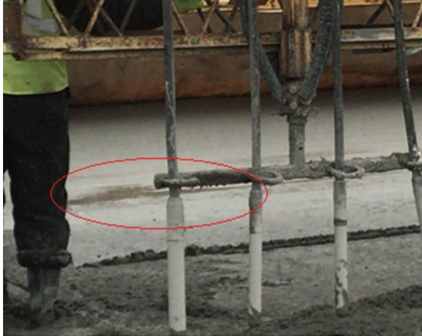
Figure 4.44: Ponded water on the surface of the bridge deck
