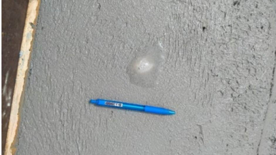
Figure 4.25: The appearance of air pockets on the concrete surface (image provided by MnDOT)
