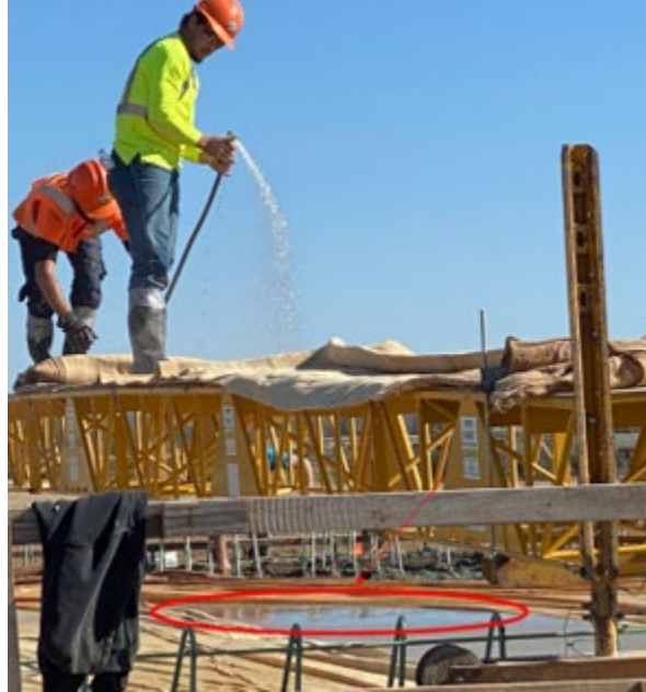
Figure 4.55: Ponding was observed on the deck
