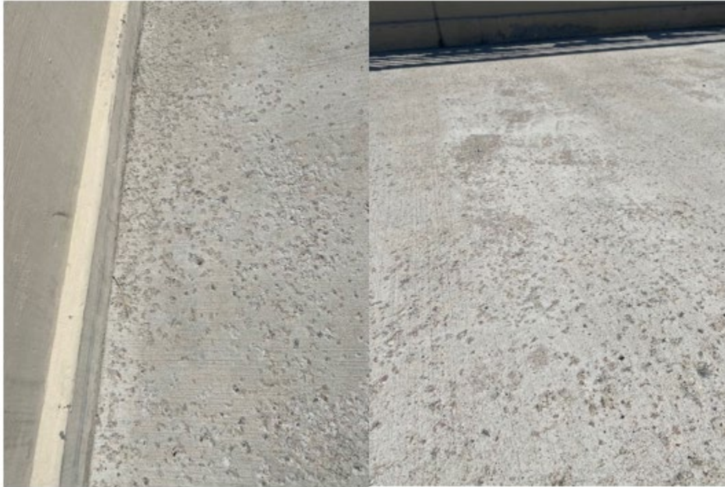
(a) (b) Figure 5.16: Scaling damage of MN-IC-LC-HPC-5 (a) near barriers; (b) a typical section for the remainder of the deck
