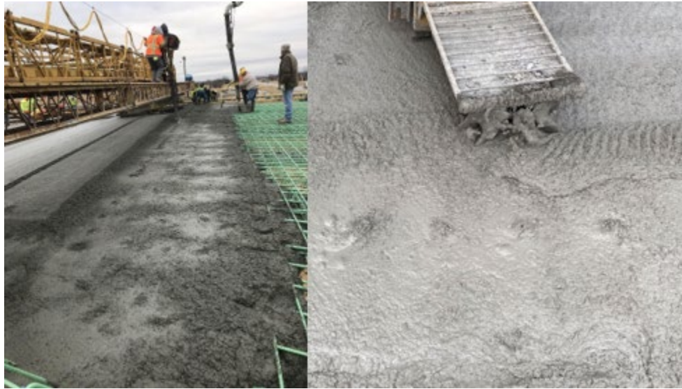
(a) (b) Figure 4.45: Holes left on the surface of the bridge deck. (a) overview; (b) close-up view
