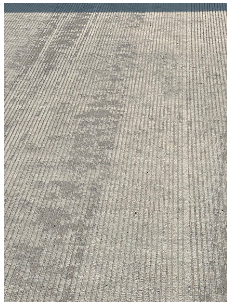
Figure 5.36: Scaling damage observed on some portions of KS-IC-LC-HPC-2
