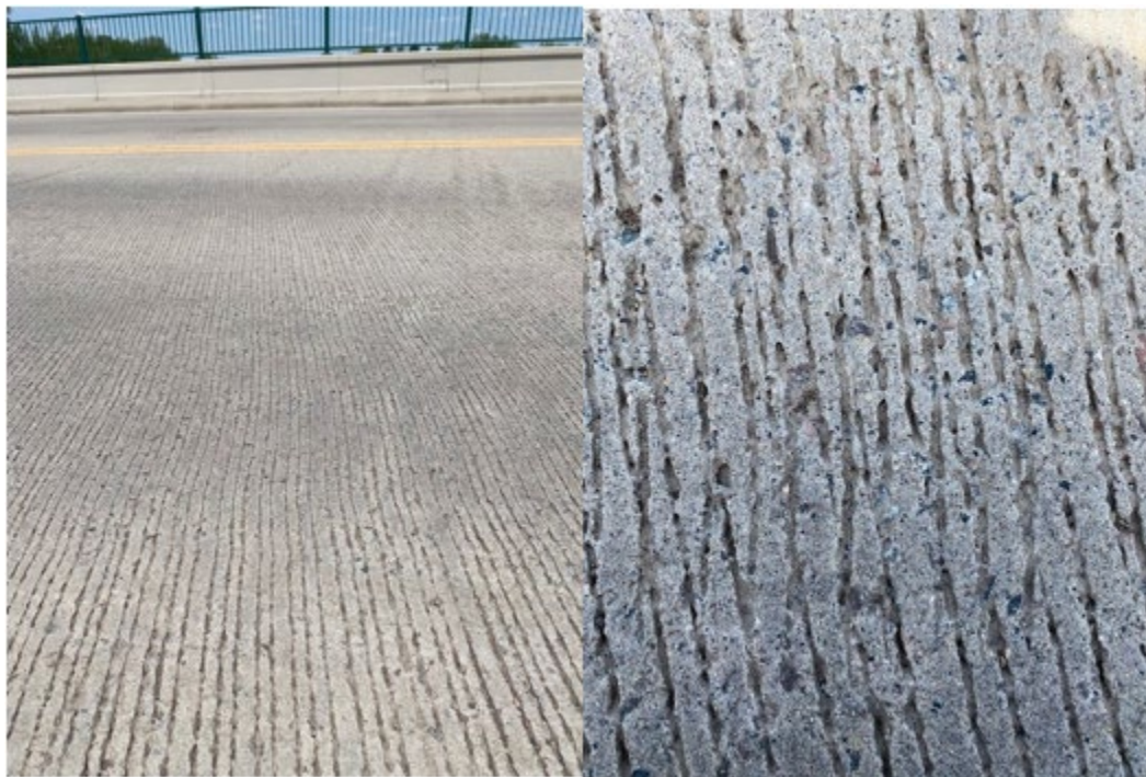
(a) (b) Figure 5.20: Poorly tining of MN-IC-LC-HPC-6 (a) an overview; (b) a close-up view
