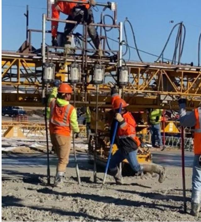
Figure 4.57: Malfunctioning of the machine-mounted gang vibrators
