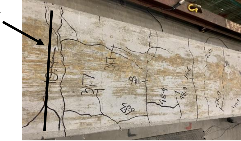
Figure 4.5: Longitudinal splitting cracks (14-f)
