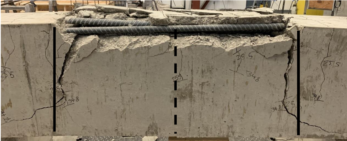
Figure E.1: Photo of 14-a after failure
