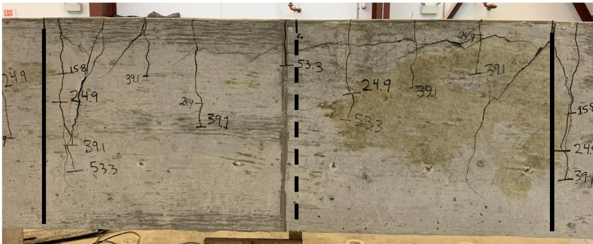
Figure E.8: Photo of 18-a after failure
