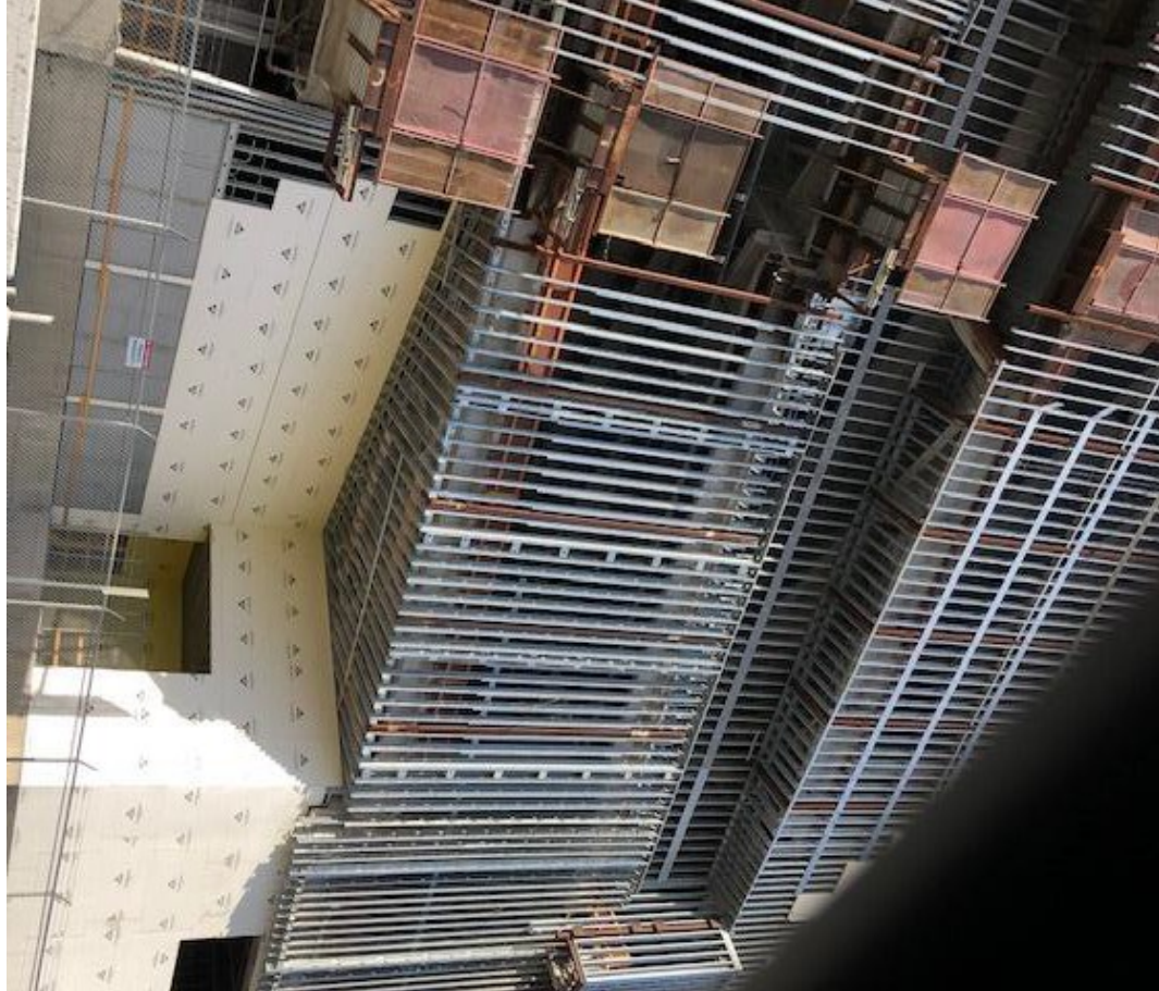
Figure 8-5: From the backside of the building it is obviously not close to completion.
