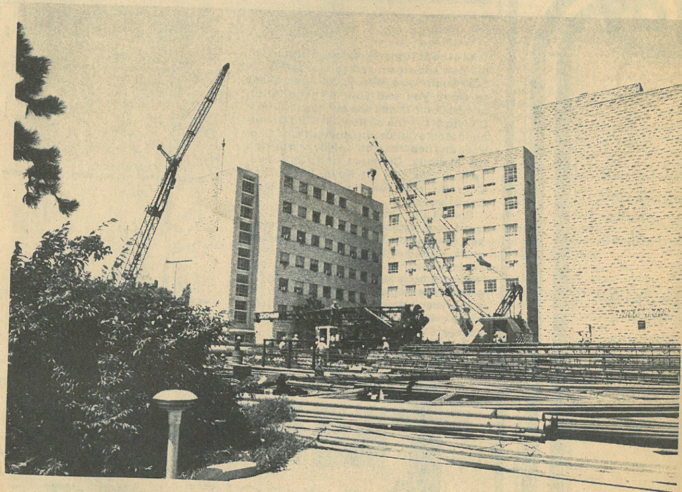
Pipes and trestles await their use in the construction of an $11.5 million addition to Malott Hall.
