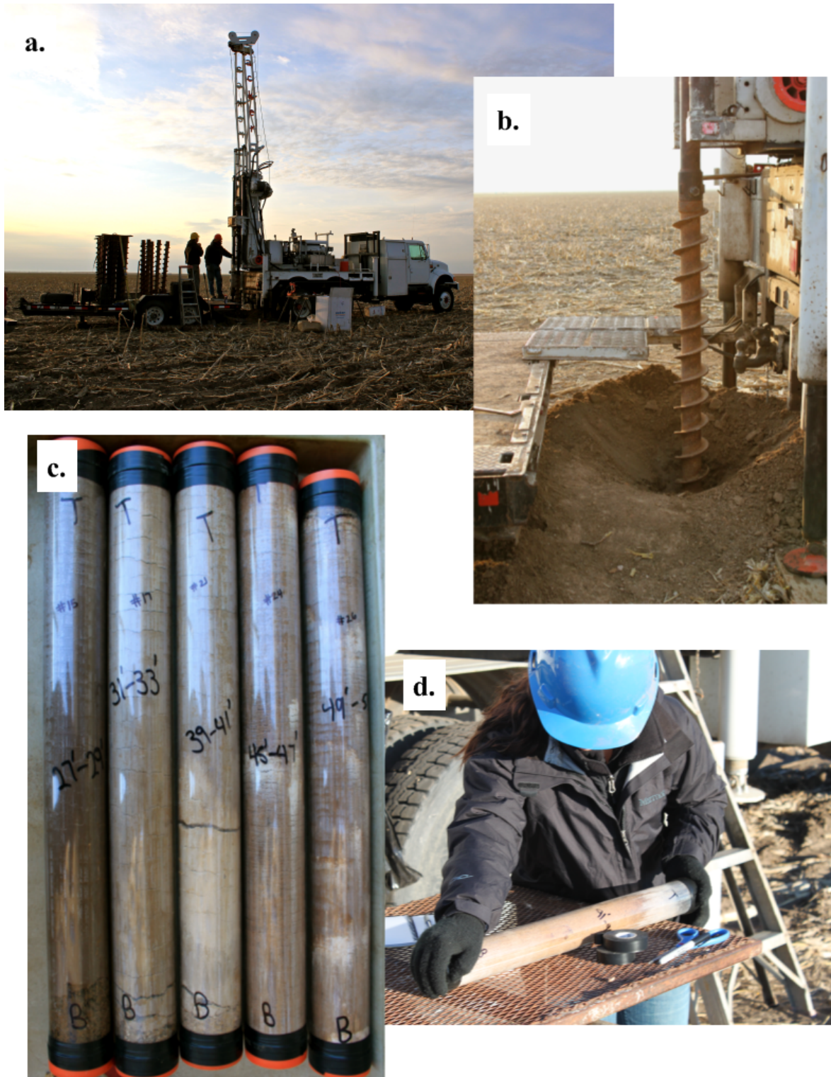
Figure 4. Photographs showing (a.) drill rig and drilling operation at the Thomas County field site on March 25, 2013, (b.) hollow-stem auger (8.3 cm diameter) in the ground at the field site, (c.) labeled sample cores tubes, and (d.) preservation of core samples by tightly sealing both ends with a rubber cap and vinyl electrical tape (to retain moisture). Photographs a., b., and c. taken by Britney S. Katz; photograph d. taken by Randy L. Stotler.
