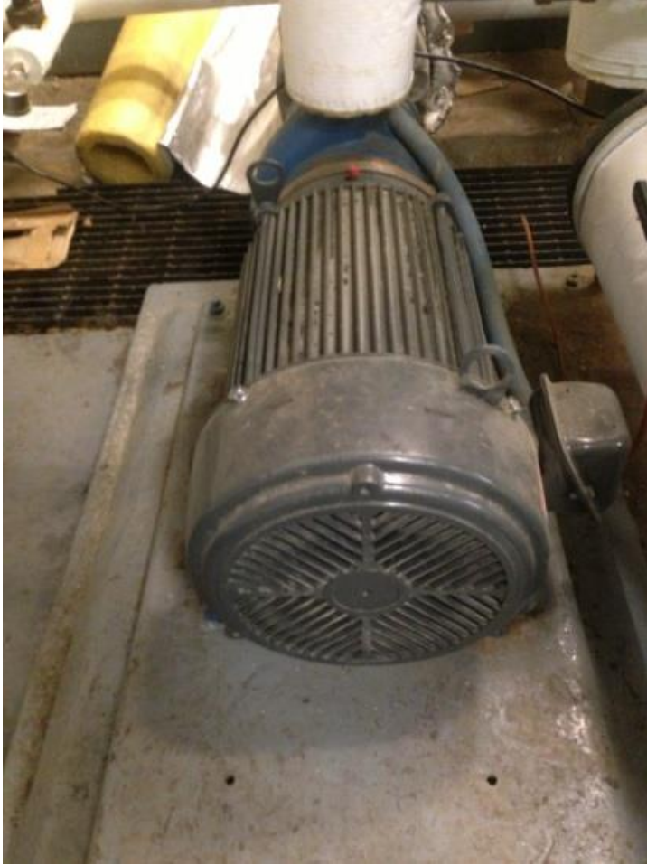
Figure 7: Worthington D-824 Centrifugal Constant Speed Pump.
